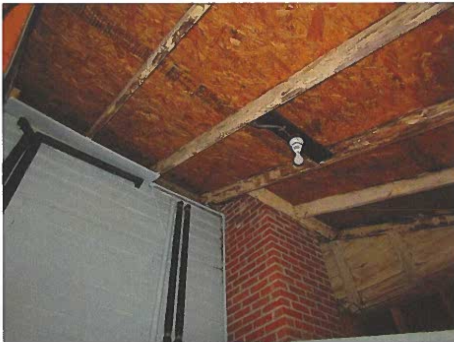
PHOTOGRAPH 10 Undersized roof rafters at the east end of the main building.
