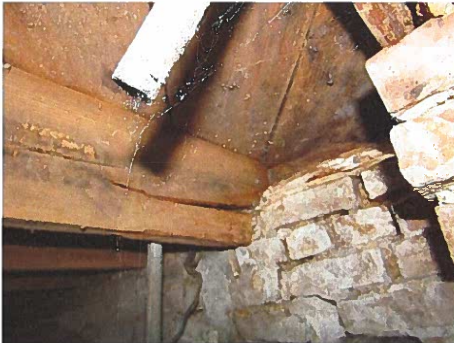
PHOTOGRAPH 16 Rotten floor joists and deteriorated brick/mortar in the crawlspace.
