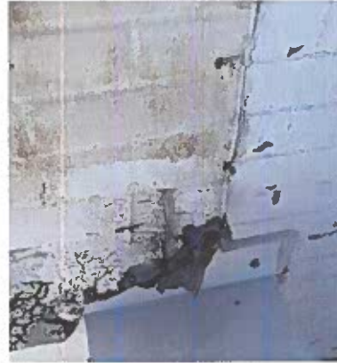
Tin paneling peeling from exterior
