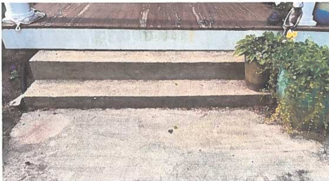
Figure 2: Existing Steps Closeup
