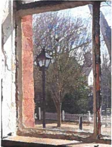
7. Detail (interior): Main hall, inappropriate repair/putty
