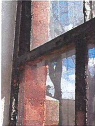
8. Detail (interior): Main hall, window sash deterioration
