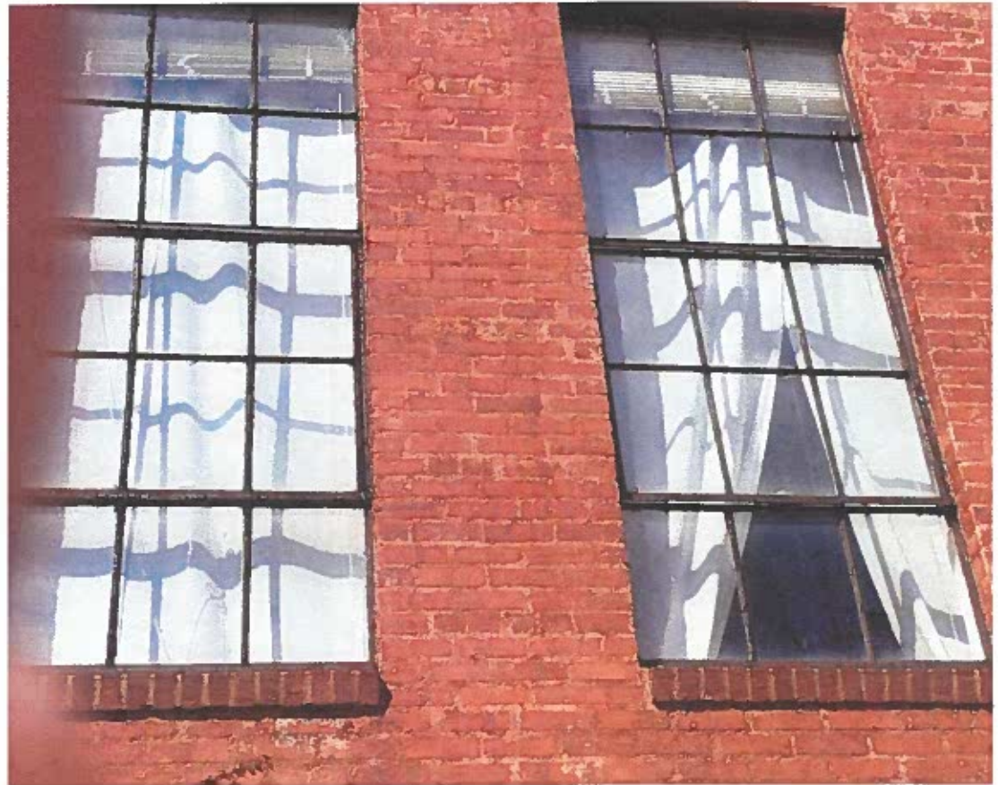
6. Detail, exterior: Main hall windows showing window size, rust issues, inability to close (right window)
