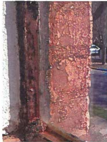
9. Detail (interior): Main hall, no putty, window sash deterioration
