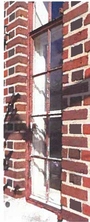
10a/b. Detail (exterior): Peeling paint, rust
