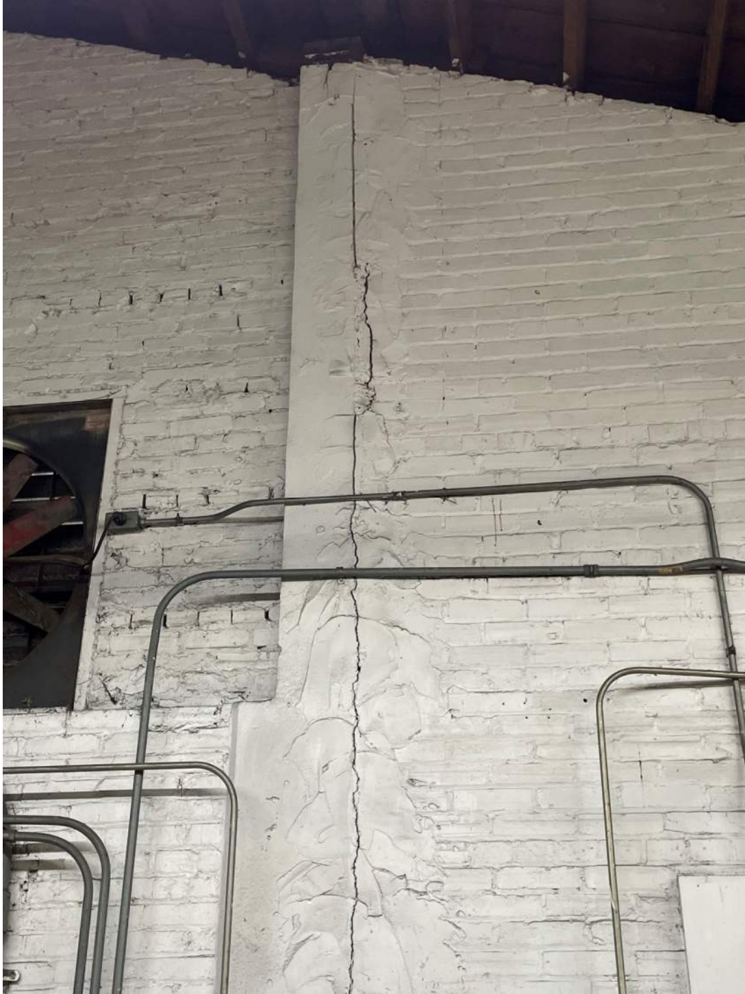
Photograph No. 11: Large Open Crack Through Existing Multi-Wythe Brick Wall
