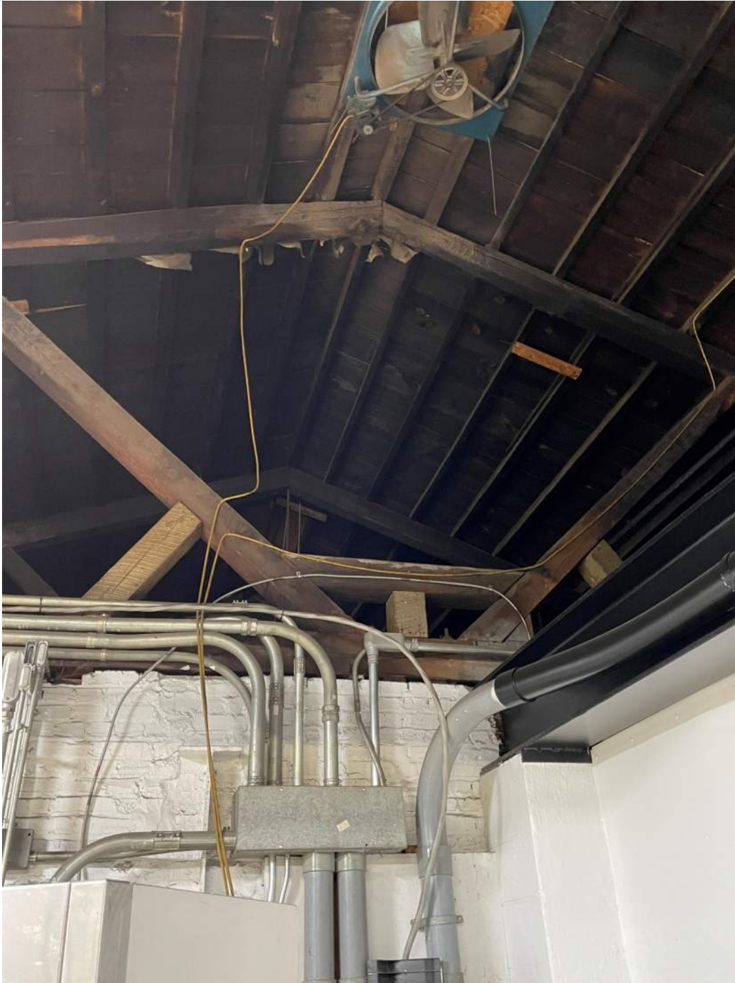
Photograph No. 7: Retrofitted Existing Wood Truss without Vertical Tension Member Between Top & Bottom Chords. Additionally, Improper Connections of Reinforcing Members that were Added.
