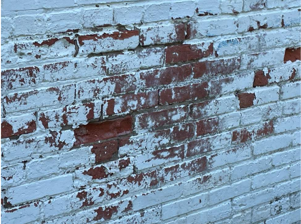
Photograph No. 14: Exterior Brick Wall & Existing Coating Delamination
