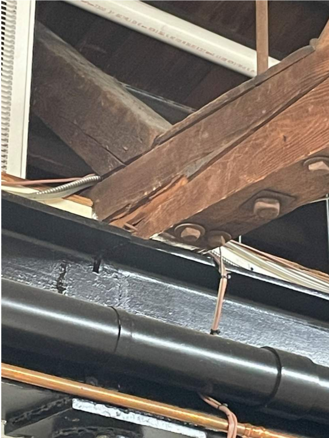
Photograph No. 8: Bottom Chord Wood Splitting at Bearing End
