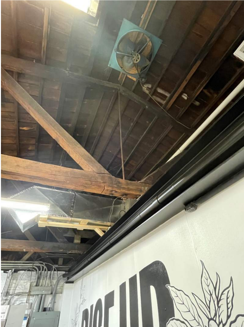
Photograph No. 4: Existing Truss with Tension Rod & Splitting of Wood at Bottom Chord
