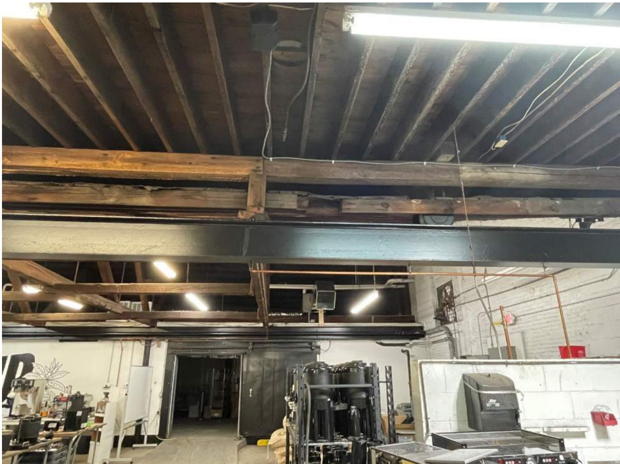
Photograph No. 16: Existing Roof Structure Transition from Addition to Original Building. Missing Structural Ties at Connections from Existing Wood Beams to Rafters & Steel Beam
