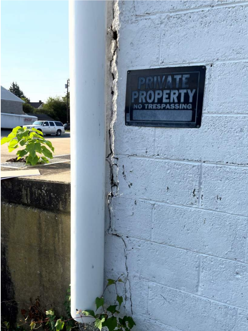
Photograph No. 22: Addition CMU Wall Cracking
