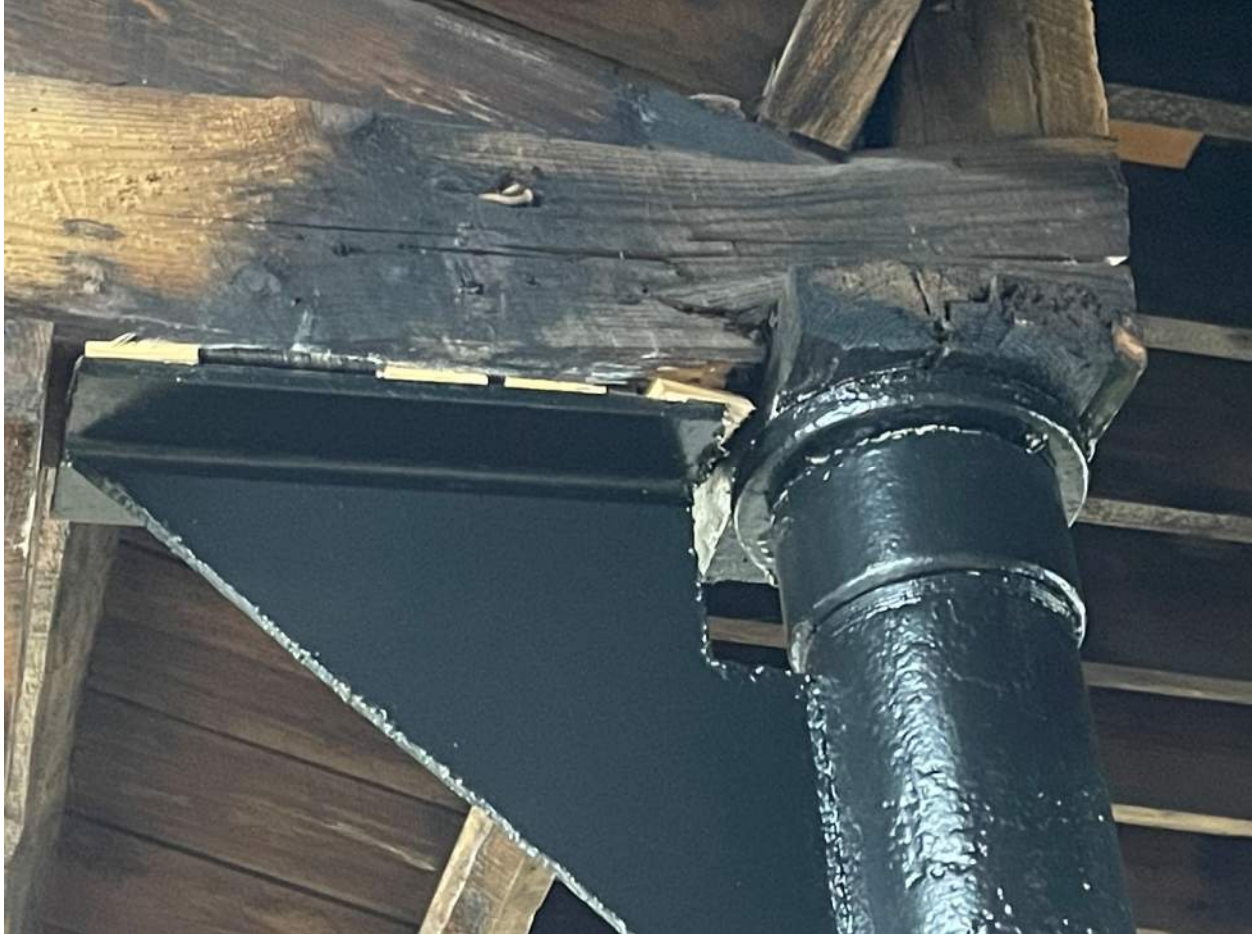
Photograph No 2: Delamination at Bearing End of Timber Truss
