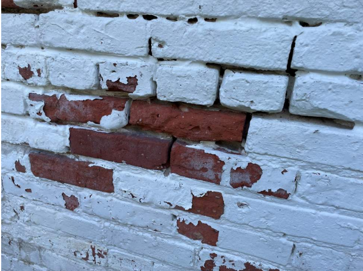
Photograph No. 13: Exterior Brick Wall & Existing Coating Delamination
