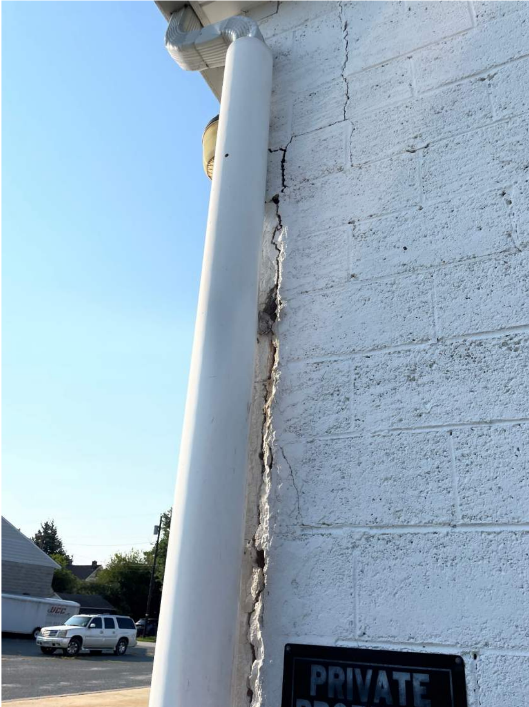
Photograph No. 21: Addition CMU Wall Cracking
