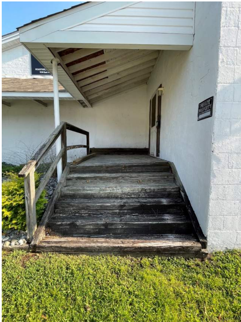
Photograph No. 25: Front Entrance Deck & Railing Delamination
