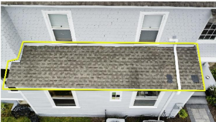
Existing architectural shingle roof with active leak
