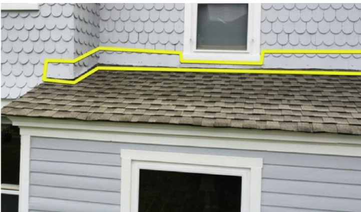
Area where flashing to be addressed, new flashing as needed will not alter existing flashing or siding
