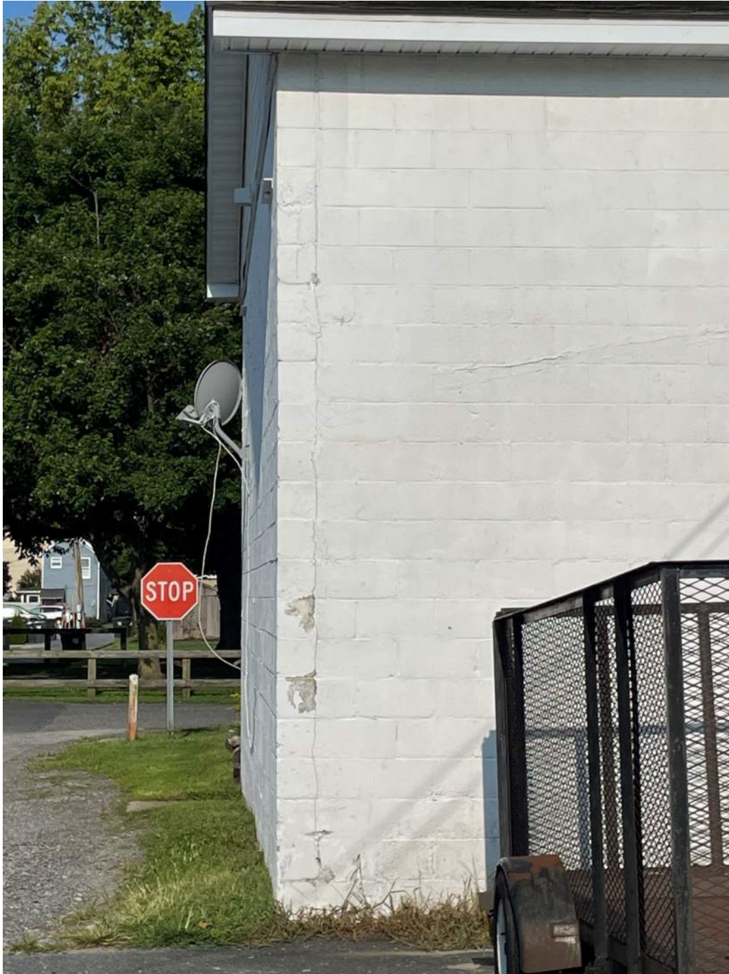
Photograph No. 24: Addition CMU Wall Cracking
