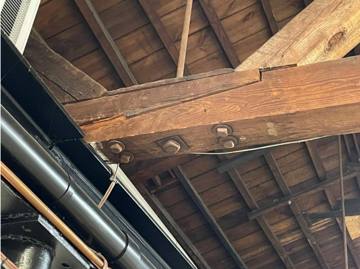
Photograph No. 6: Loose Connections at Existing Bottom Chord Splice Location Along with Damage to Bottom Chord & Splitting of Diagonal Wood Member
