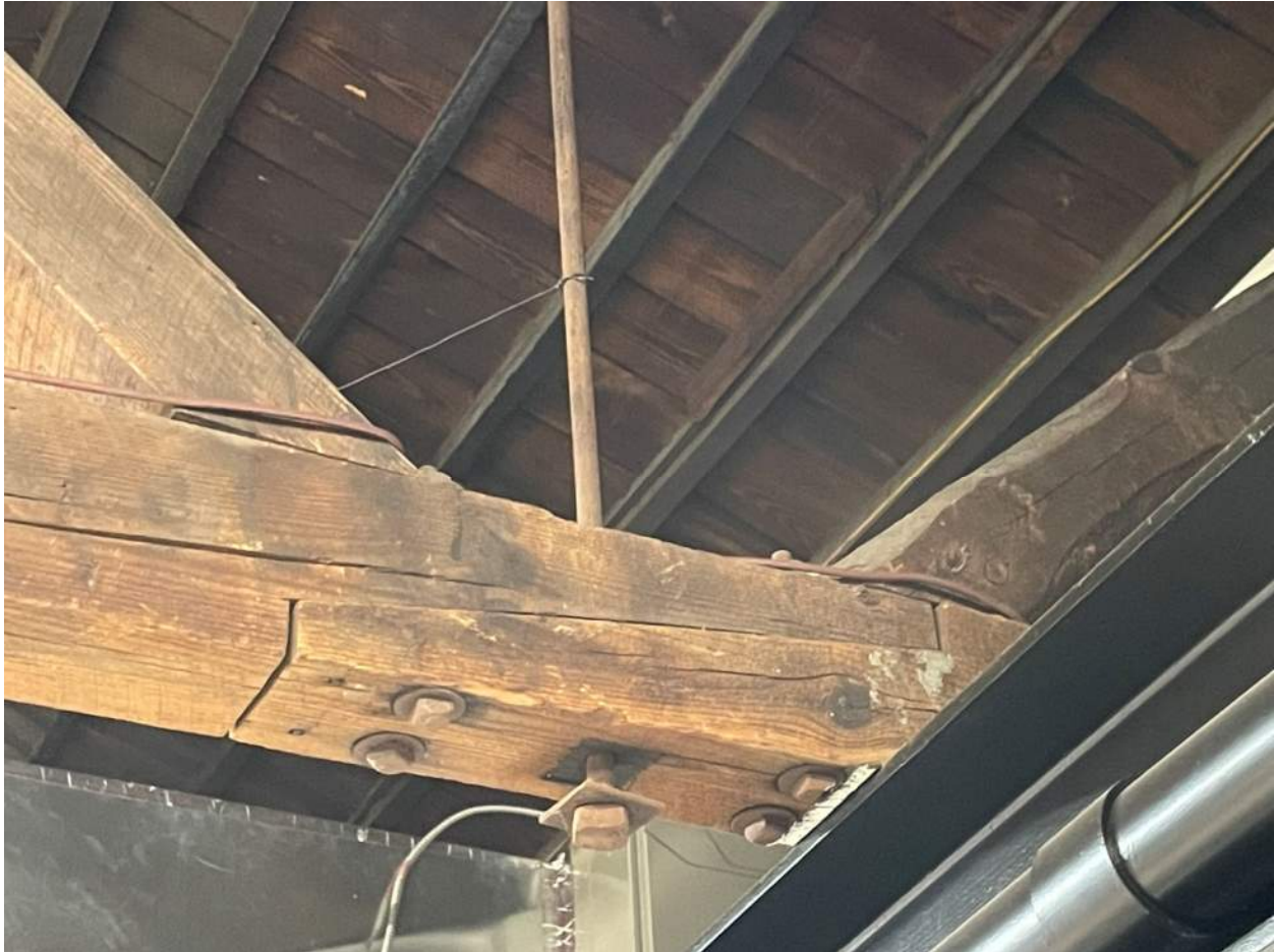
Photograph No. 5: Truss Chord Splitting at Splice Location & Loose Connections of Tension Rod to Bottom Chord
