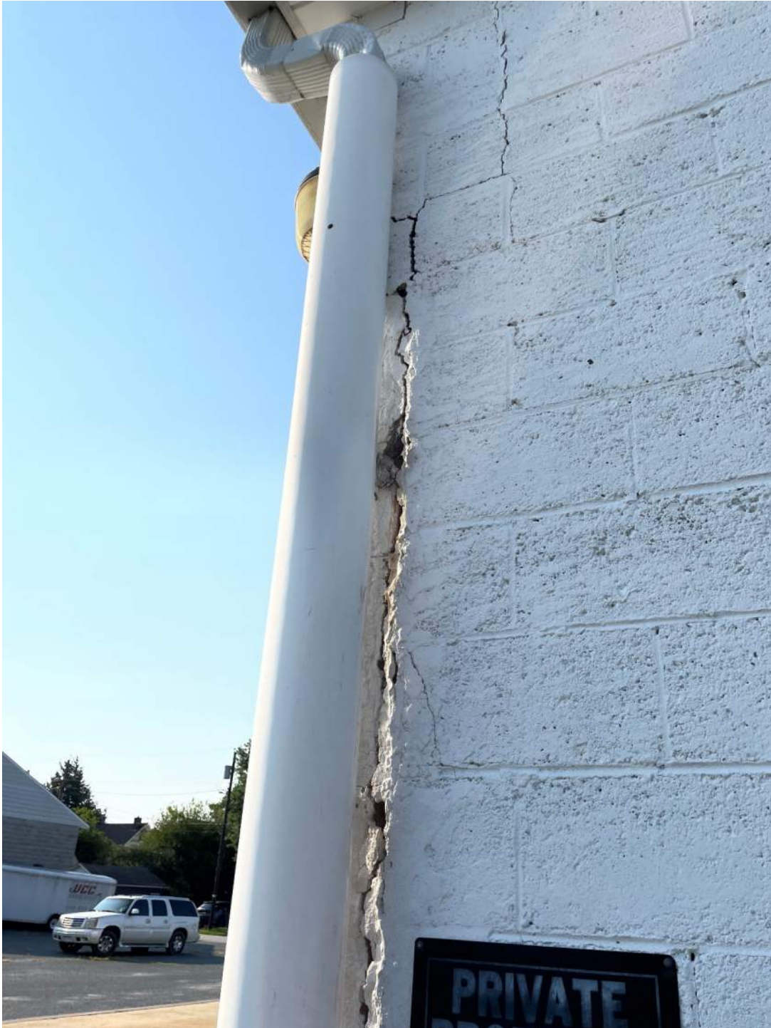
Photograph No. 21: Addition CMU Wall Cracking
