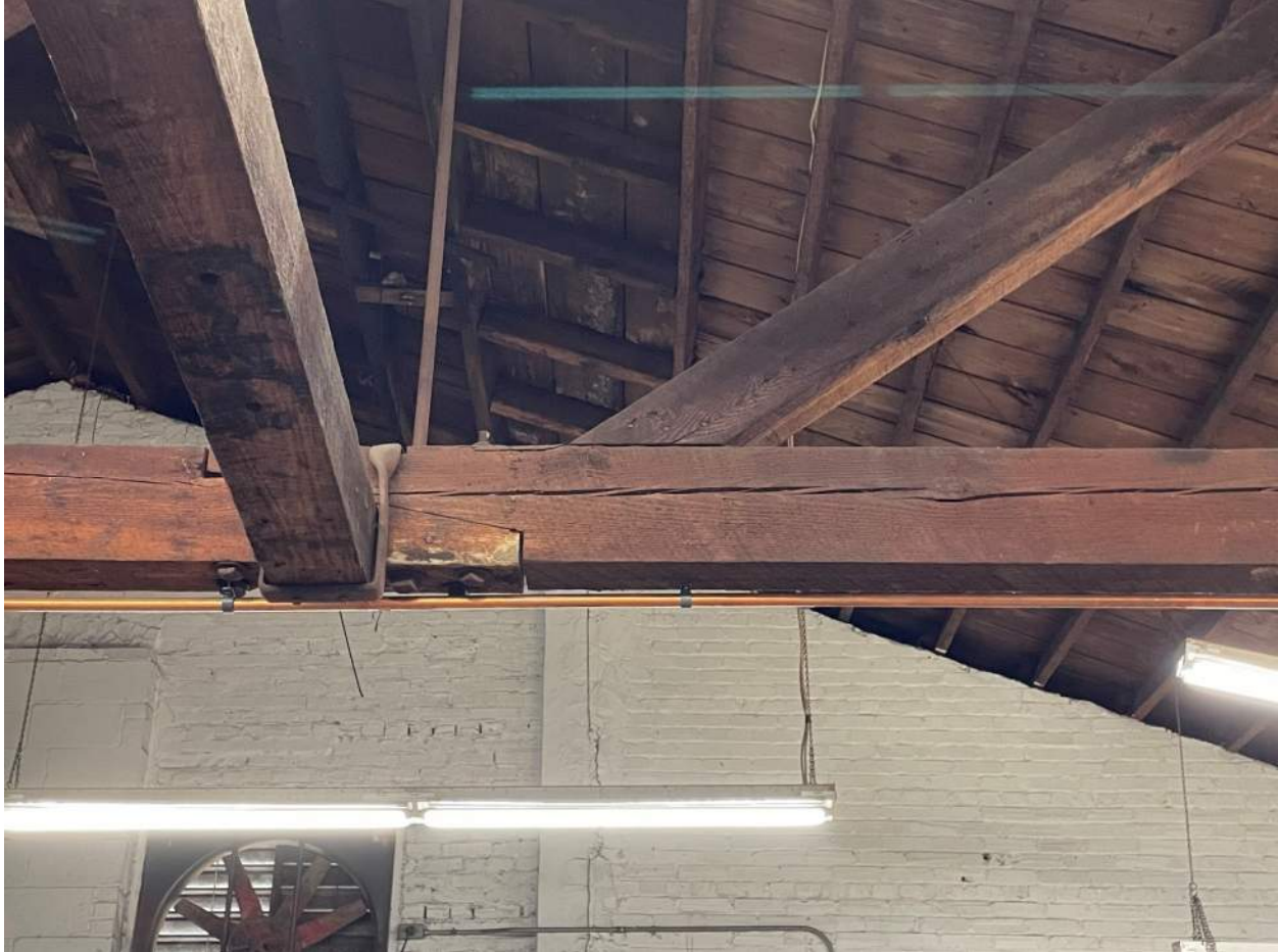
Photograph No. 9: Continuous Bottom Chord Wood Splitting Through the Bottom Chord Splice Location
