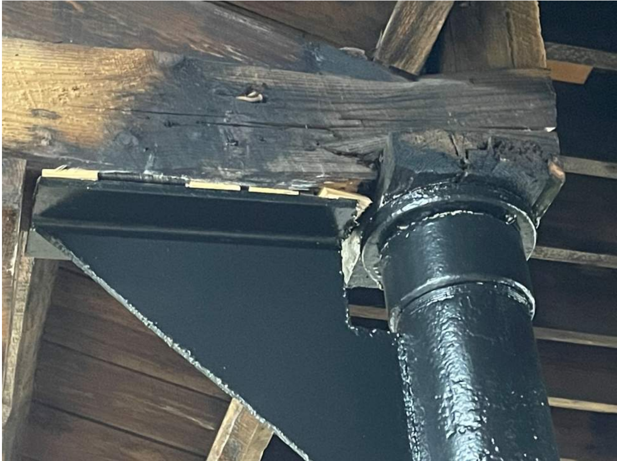
Photograph No 2: Delamination at Bearing End of Timber Truss
