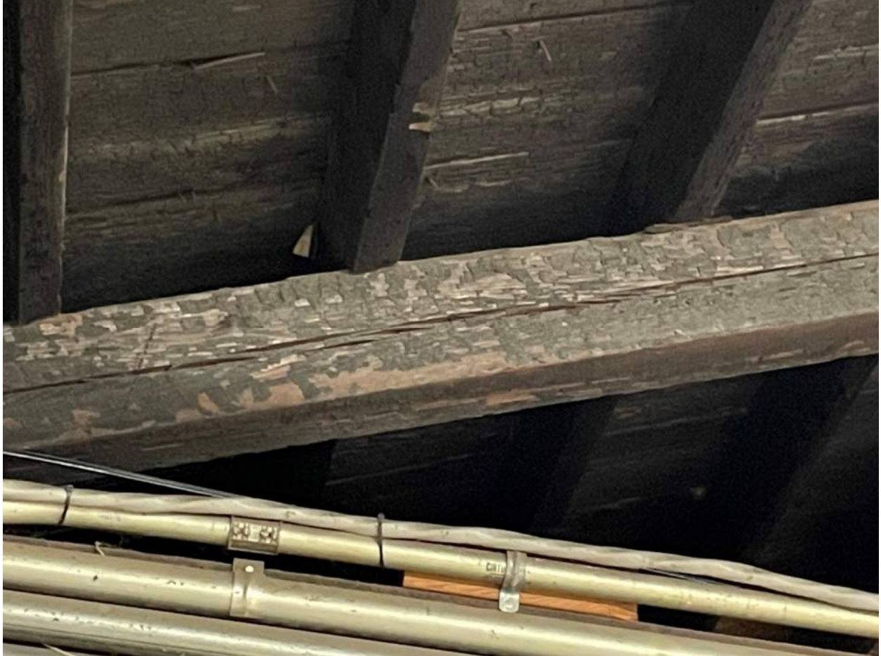
Photograph No. 3: Wood Splitting at Truss Top Chord
