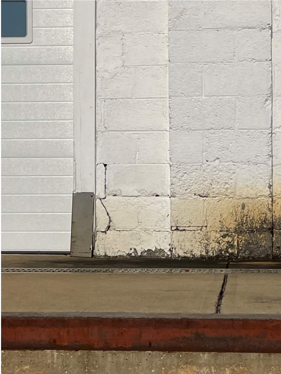
Photograph No. 23: Addition CMU Wall Cracking
