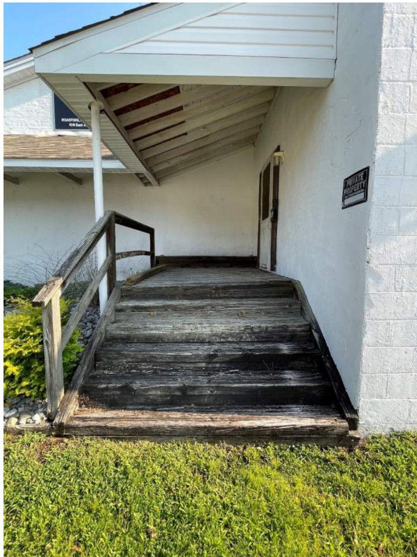
Photograph No. 25: Front Entrance Deck & Railing Delamination
