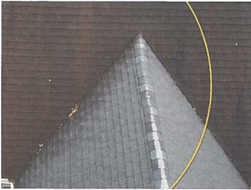
This is the second story and you can see severe granule loss on the ridge caps.
