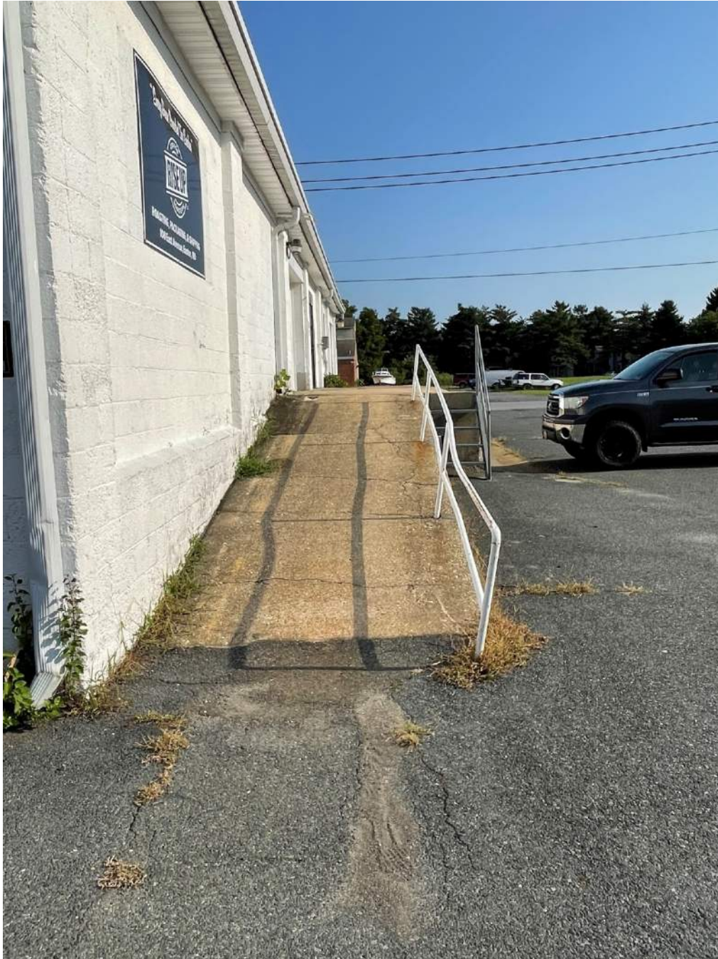
Photograph No. 26: Loading Dock Railing Corrosion & Failure
