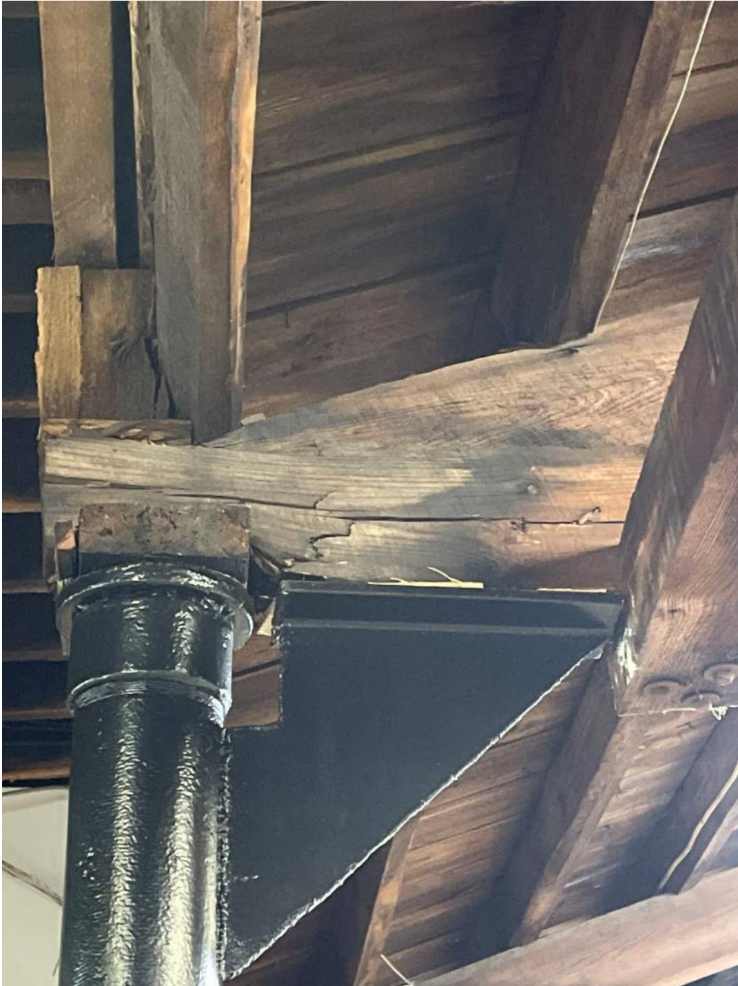
Photograph No. 10: Truss Bearing Failure / Crushing / Splitting of Truss Bottom Chord
