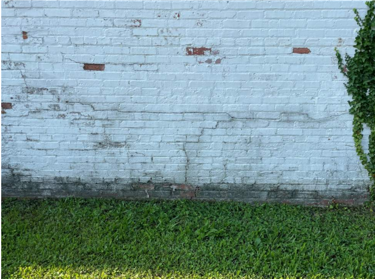
Photograph No. 15: Exterior Brick Wall Horizontal, Step, & Vertical Cracking. Horizontal Cracking Occurring at Level of Interior Floor Slab. Observed Rotation of Existing Brick Wall from Exterior Grade Up to Existing Horizontal Crack.
