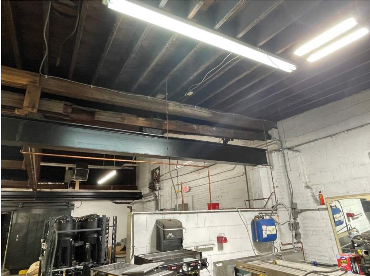
Photograph No. 17: Existing Roof Structure Transition from Addition to Original Building. Missing Structural Ties at Connections from Existing Wood Beams to Rafters & Steel Beam
