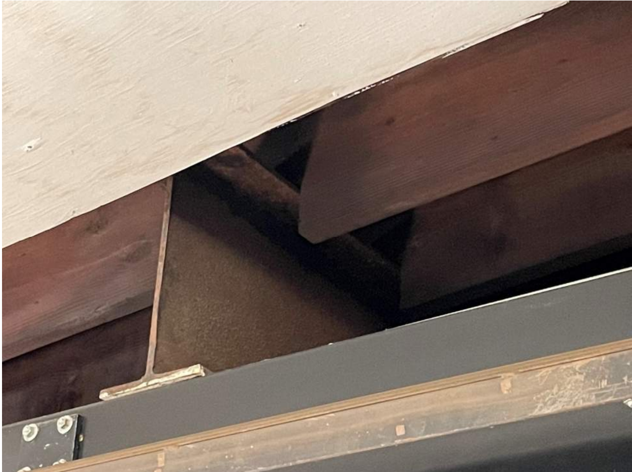
Photograph No. 19: Existing Roof Rafters Cut at Bearing End at Steel Beam Location with Not Rafter Hangers
