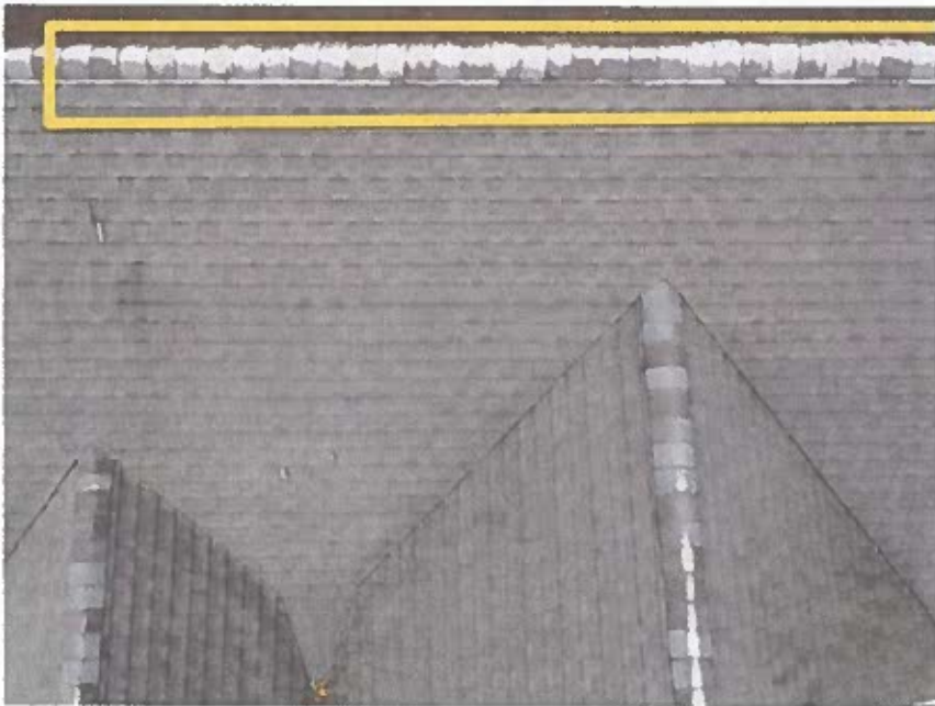
This is the main ridge of the roof with severe granular loss.
