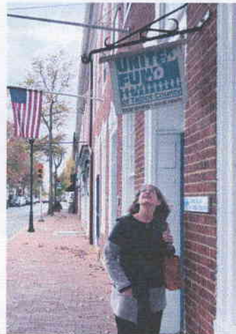
Bracket to be reworked for level and re-mounted for 8' clearance below sign
