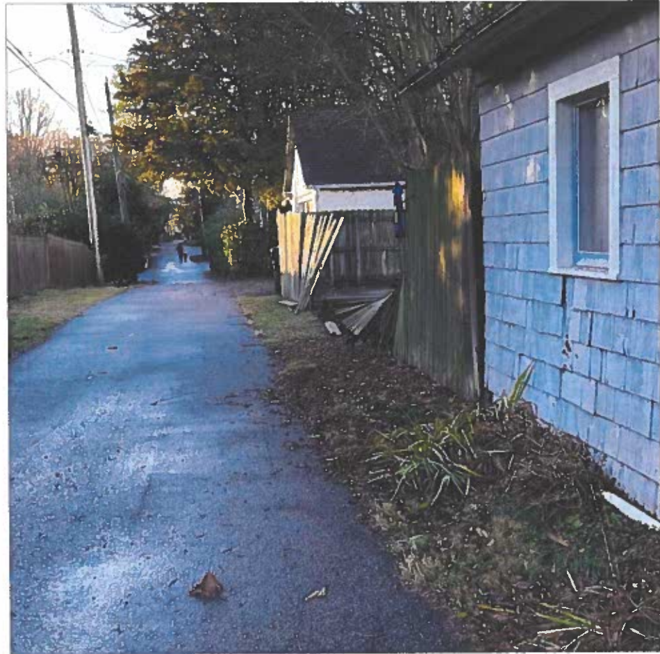
Existing Damaged Fence
