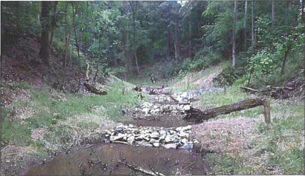
PHOTO 1. EXAMPLE PROJECT WITH COBBLE WEIRS WITH POOLS TO ATTENUATE STORM FLOWS HANDLES LARGE VOLUMES OF WATER AT STEEP DROPS.
