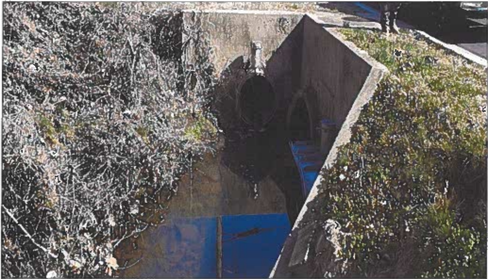
PHOTO 1. EXTREME INCISION IMMEDIATELY DOWNSTREAM OF PIPE. INCISION IS LIKELY DUE TO SHEET RUNOFF FROM SURROUNDING IMPERVIOUS SURFACES.
