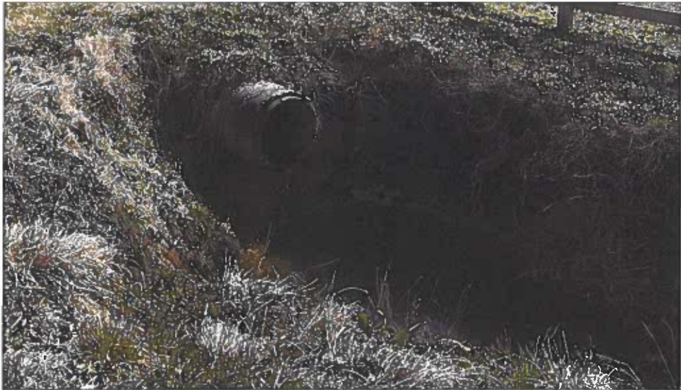
PHOTO 1. EXTREME SCOUR UNDER PIPE EXHIBITS FLOODPLAIN DISCONNECTION AND INCISION.
