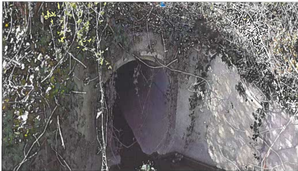
PHOTO 4. ROAD CULVERT AT DOWNSTREAM EXTENT IS PROVIDING BACKWATER.
