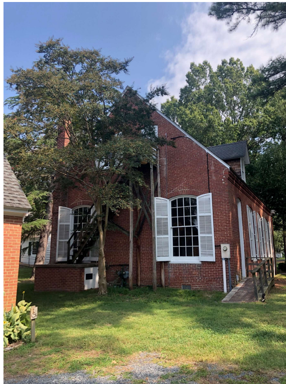
Rear (West) Elevation –Showing noncompliant 2 nd floor exit stairs
