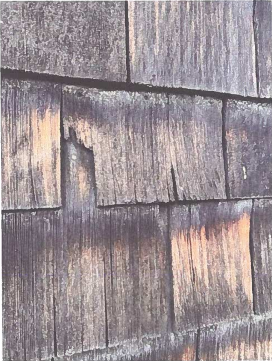
Existing worn cedar shingles (1)
