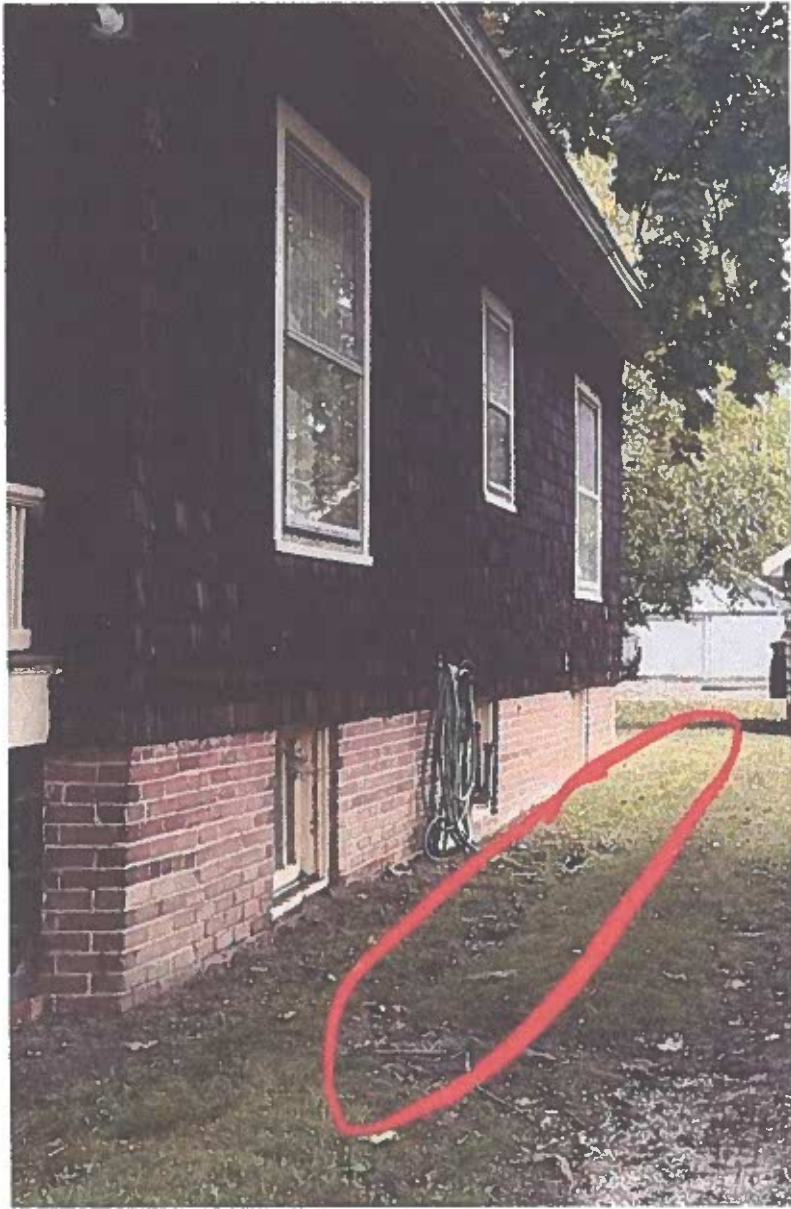
Ground impacted by need for gutters
