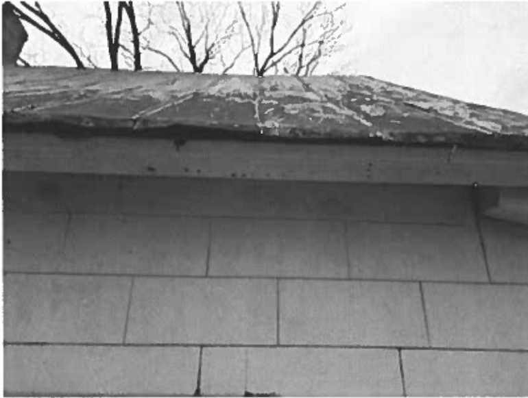
Parts of this roof have pulled up from the purlins
