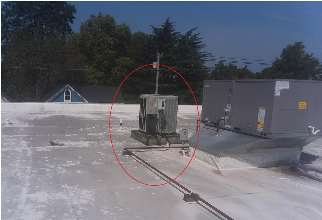
Existing RTU-3 to be replaced
