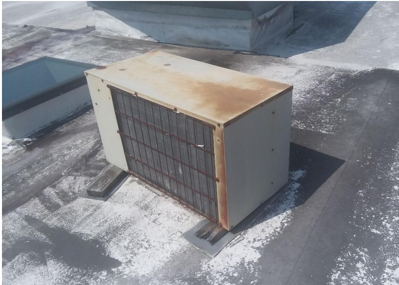
Existing ODU-1 to be replaced
