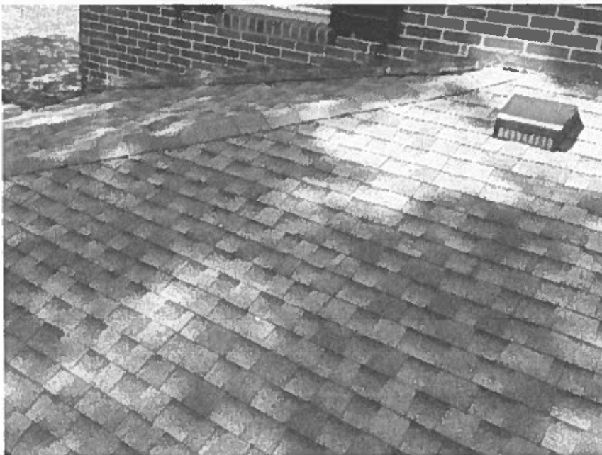
This slope of shingles is newer than the rest of the roof. It is in much better condition but would still need to be replaced to tie in to the flat roof section.
