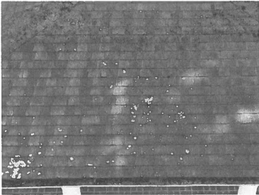
More examples of granular loss.
