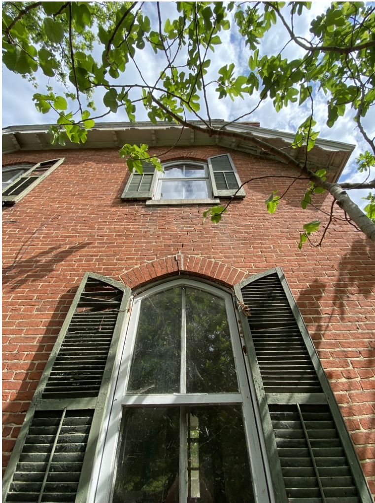
10 STRESS FRACTURE - BRICK
