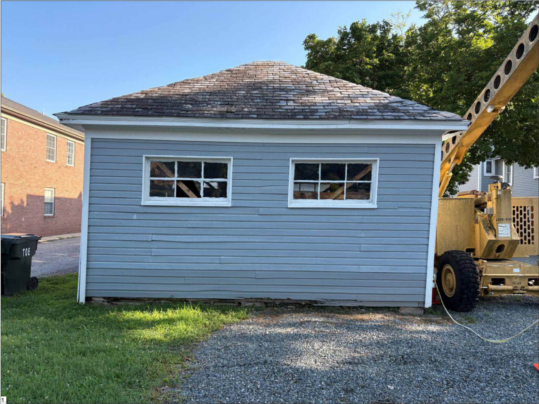
SOUTH ELEVATION ROOF NEEDS TO BE REPLACED, BUILDING IS LEANING TO THE EAST, DAMAGE TO WINDOWS, SOFFIT, FACIA AND SILL PLATE.
