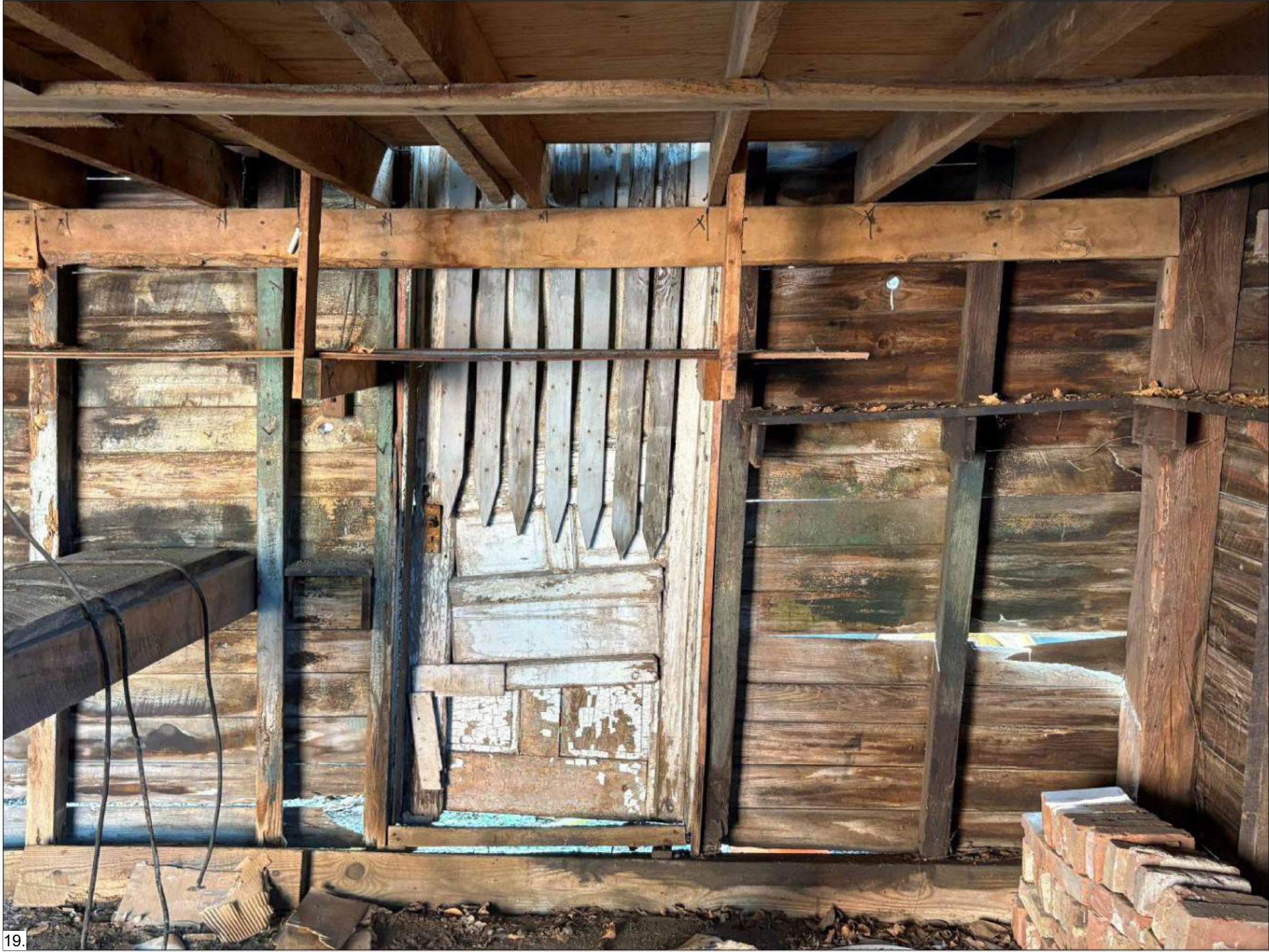
19. INTERIOR EAST WALL STUDS ARE LEANING, EXISTING DOOR NEEDS REPLACEMENT, NEW LEDGER BOARD HAS BEEN INSTALLED TO STABILIZE STRUCTURE
