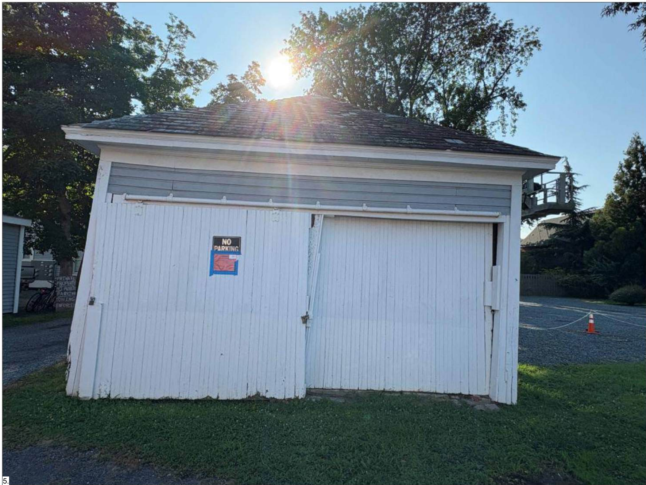
WEST ELEVATION EXTREME TILTING OF THE BUILDING DUE TO ROTTED SILL PLATES AND OVERALL DECAY TO WOOD STRUCTURAL MEMBERS.
