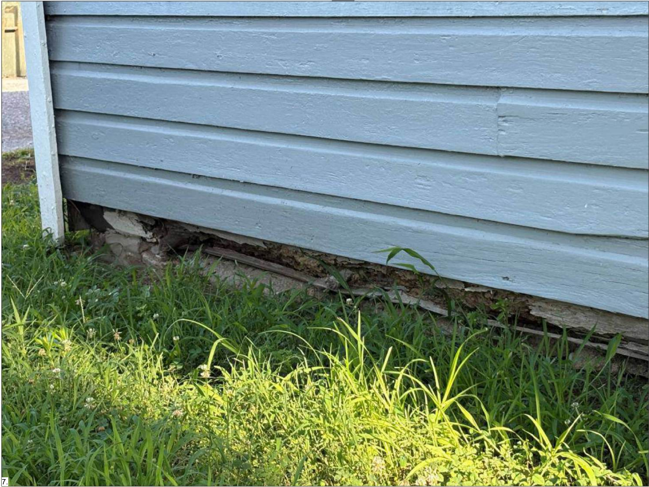
7. SOUTH SILL PLATE SEVERE TERMITE DAMAGE AND ROT CAUSING THE BUILDING TO LEAN, UNCLEAR ABOUT INTEGRITY OF FOUNDATION BUT INTERIOR SLAB HAS CRACKING
