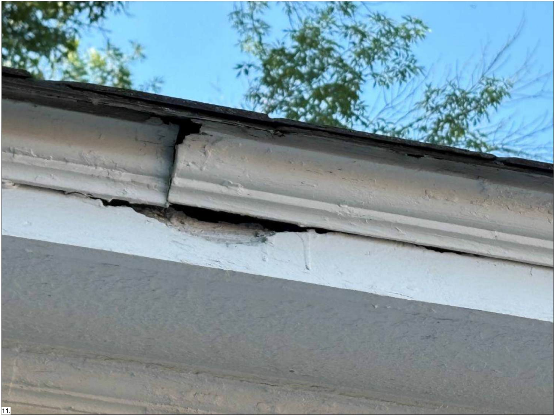
11. CROWN MOLDING DETAIL FACIA AND CROWN MOLDING NEED REPLACEMENT DUE TO EXTENSIVE ROT AND RODENTS
