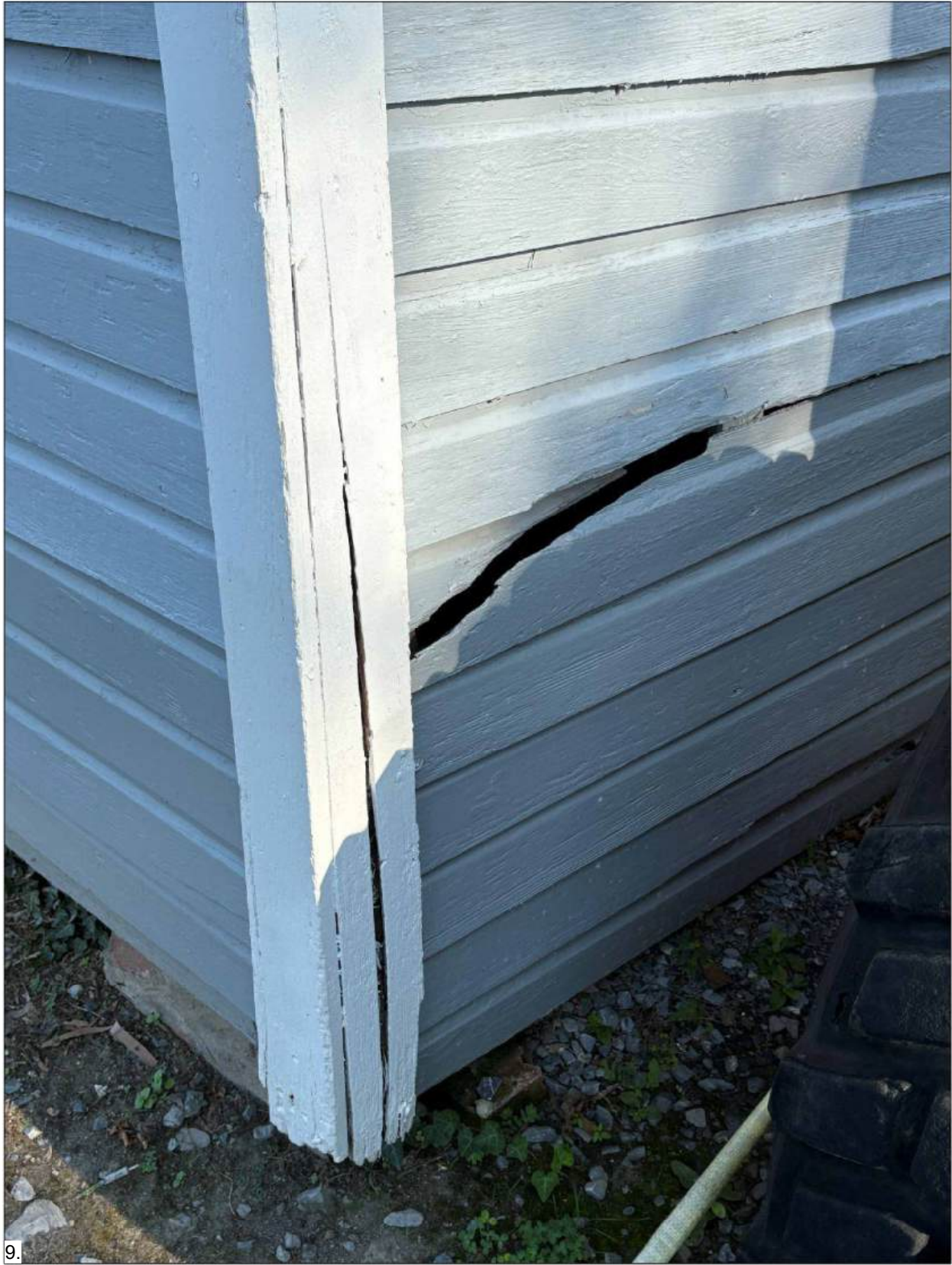
9. SOUTHEAST CORNER DAMAGE AT CORNER BOARDS AND SIDING, SIDING IS RESTING ON THE GROUND IN SOME AREAS
