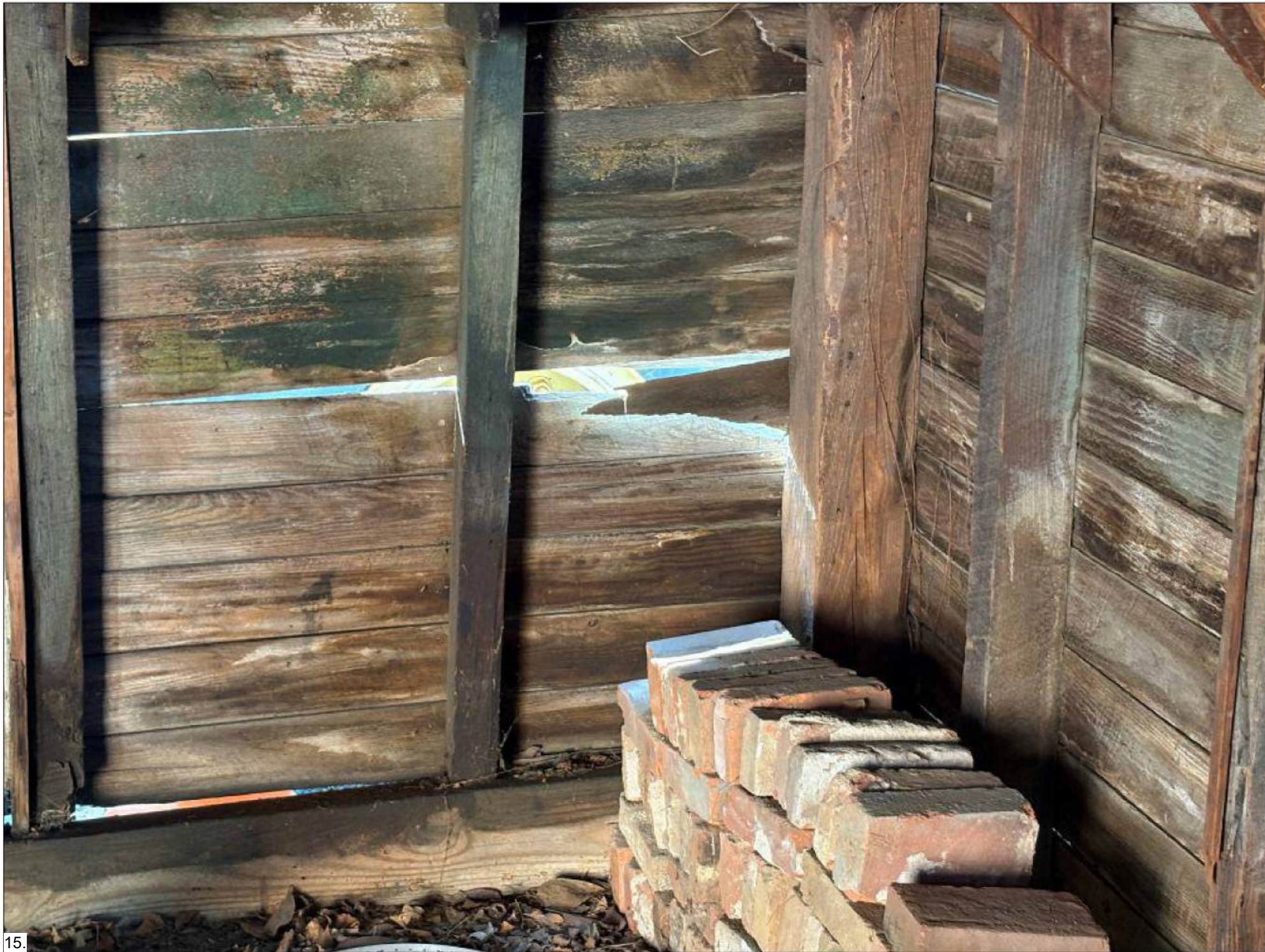
15. INTERIOR SOUTHEAST CORNER SIDING NEEDS REPLACEMENT
