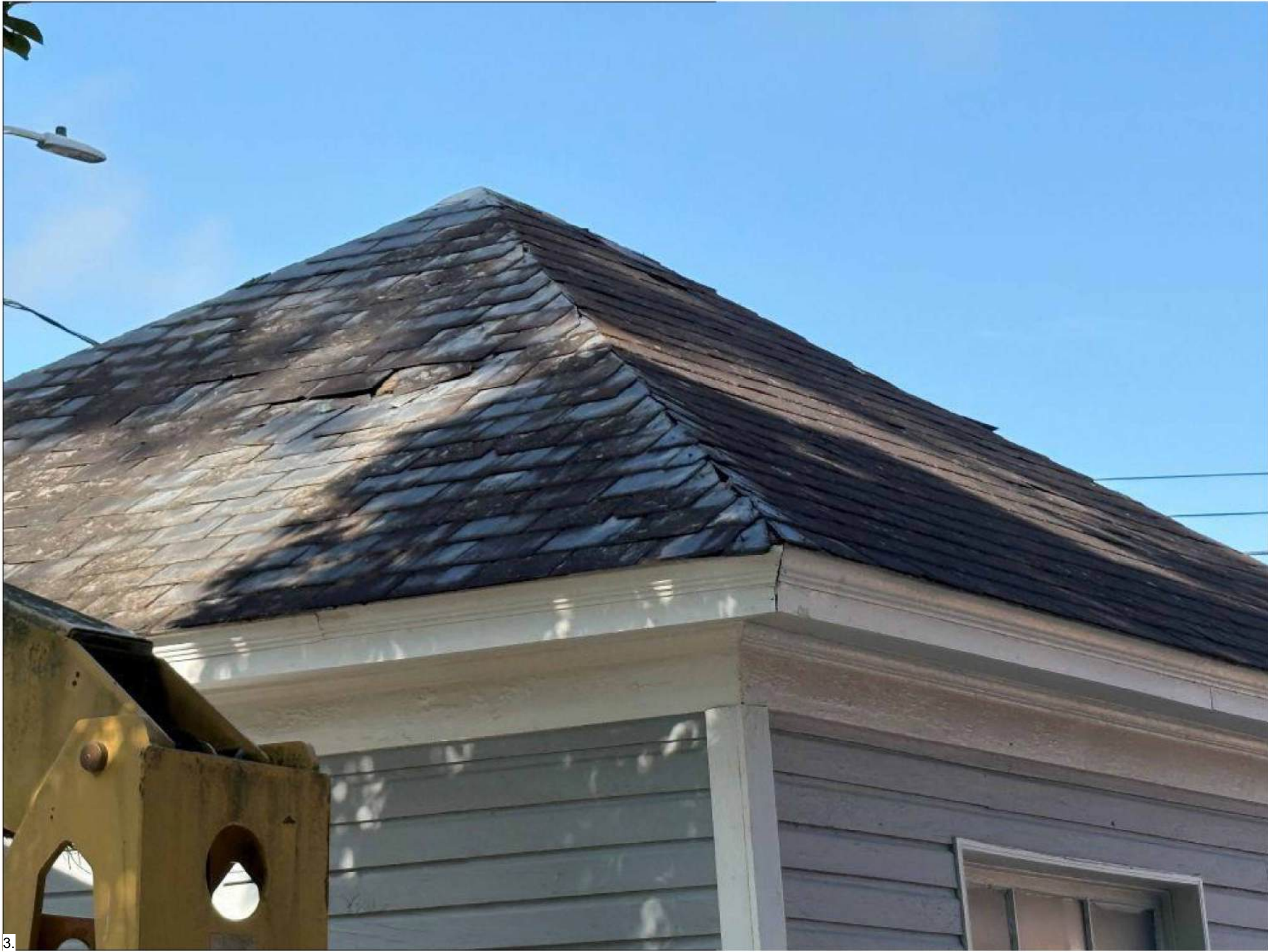
NORTHEAST CORNER ROOFING SLATE IS COMPROMISED AND ROOFING BOARDS HAVE LARGE OPENINGS DUE TO DECAY AND MOLD.
