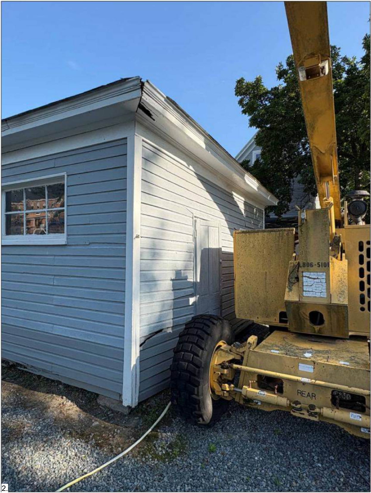
SOUTHEAST CORNER DAMAGE TO SIDING, CORNER BOARDS AND SOFFIT, SILL PLATE SHOWS ROT AND TERMITE DAMAGE.
