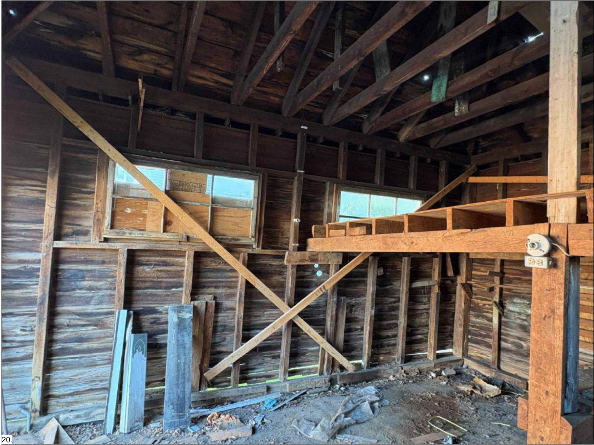
20. INTERIOR NORTH WALL ROOF RAFTERS/JOISTS SHOW MOLD AND DECAY. WALL HAS BEEN BRACED WITH 2 X 4'S TO STABILIZE STRUCTURE
