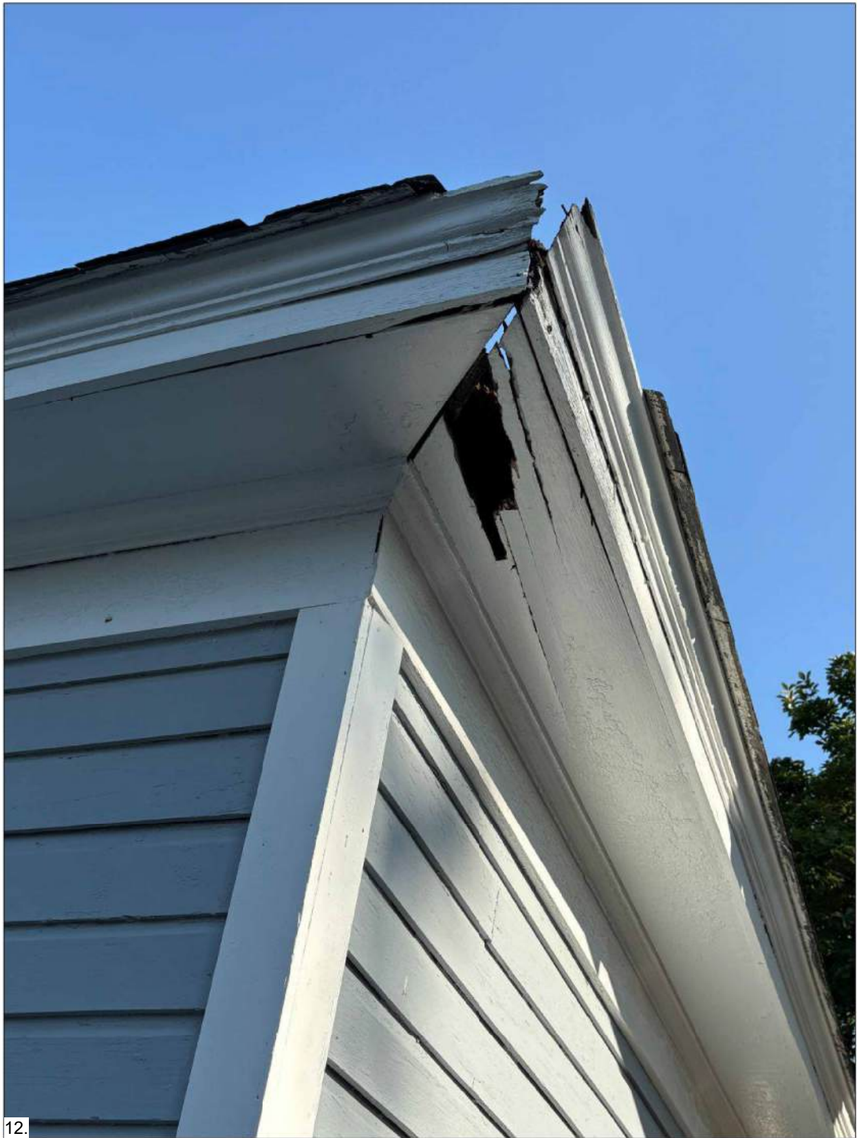
12. SOFFIT AND CROWN MOLDING DETAIL ROOFING SLATE IS MISSING AT THIS CORNER, SOFFIT, CROWN AND FACIA NEED REPLACEMENT
