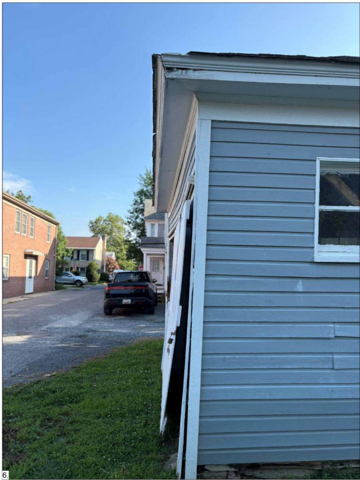
SOUTHWEST CORNER EXTREME BUILDING TILT, ROTTED SILLS AND TRIM. EVIDENCE OF SIDING BUCKLING DUE TO COMPROMISED STRUCTURE.
