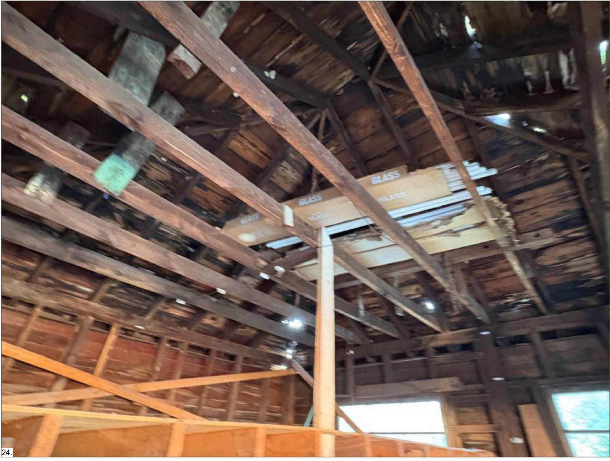
24. ROOF STRUCTURE JOISTS ARE 2 X 4 CONSTRUCTION, ROOFING BOARDS AND ROOFING SLATE SHOWS EXTENSIVE DAMAGE.
