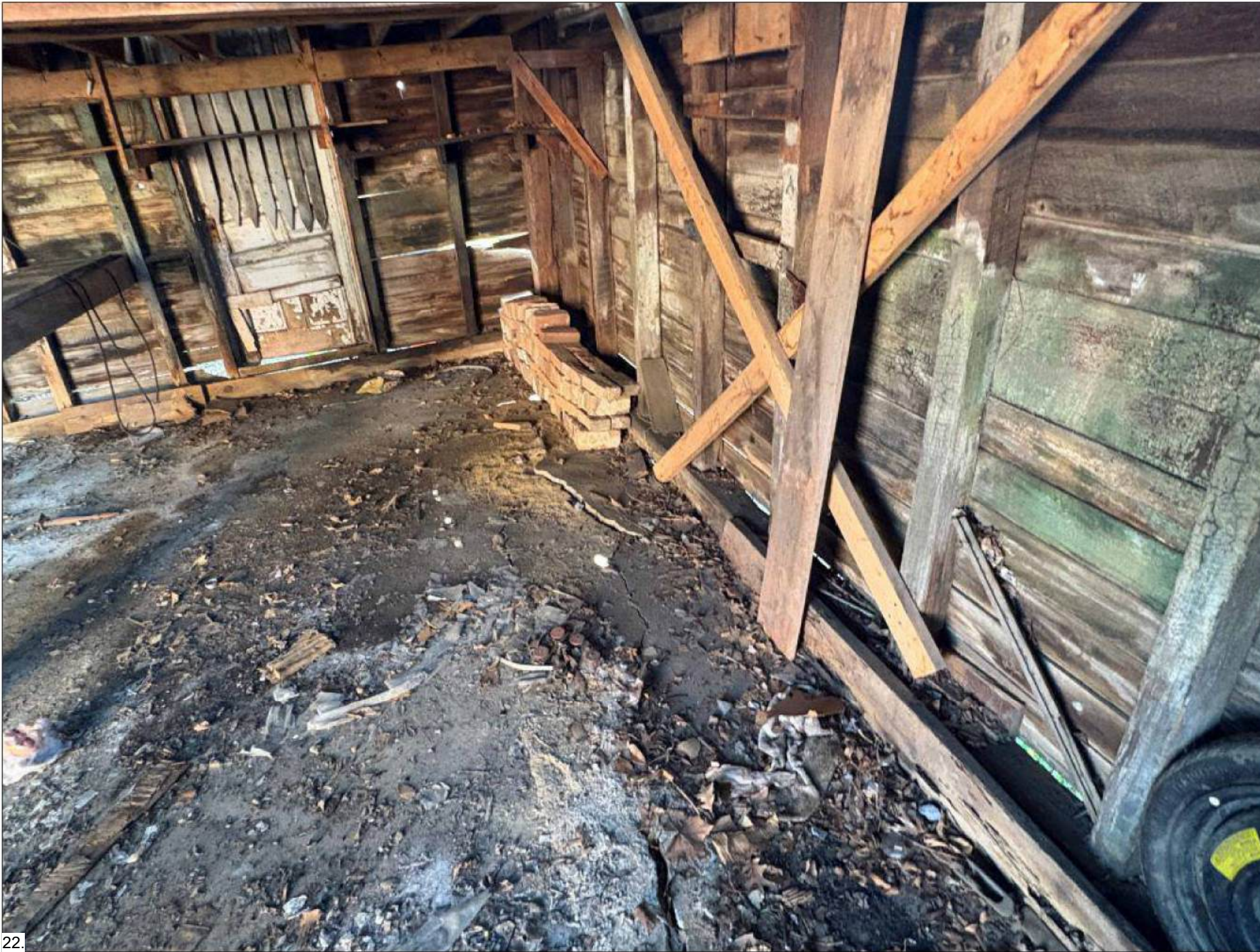
22. INTERIOR SOUTH WALL COMPROMISED SILL PLATE, AND SLAB SHOWS EXTENSIVE CRACKING
