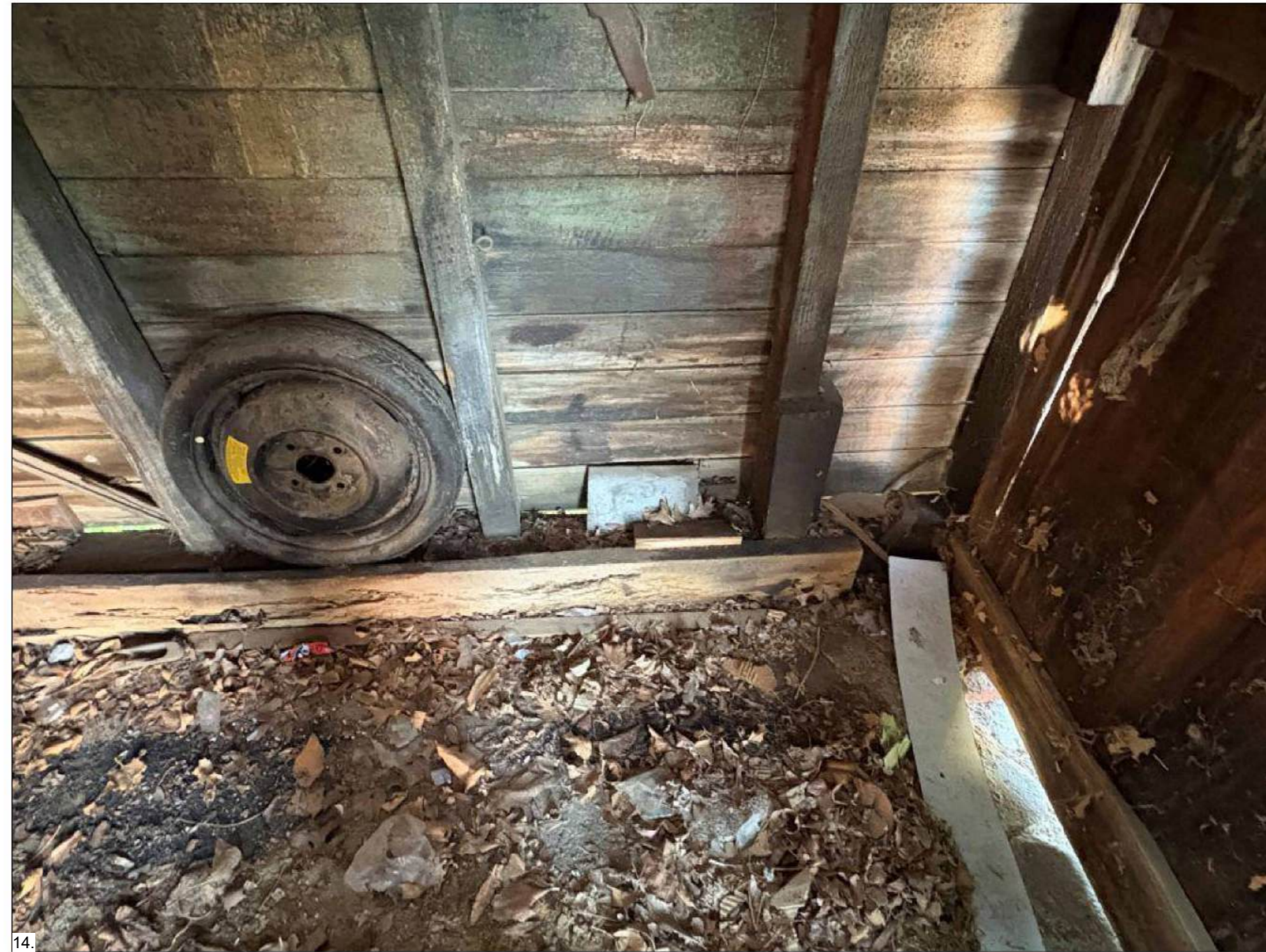
14. INTERIOR SOUTHWEST CORNER EXTENSIVE TERMITE DAMAGE AND ROT AT SILL PLATE, STUDS ARE LEANING
