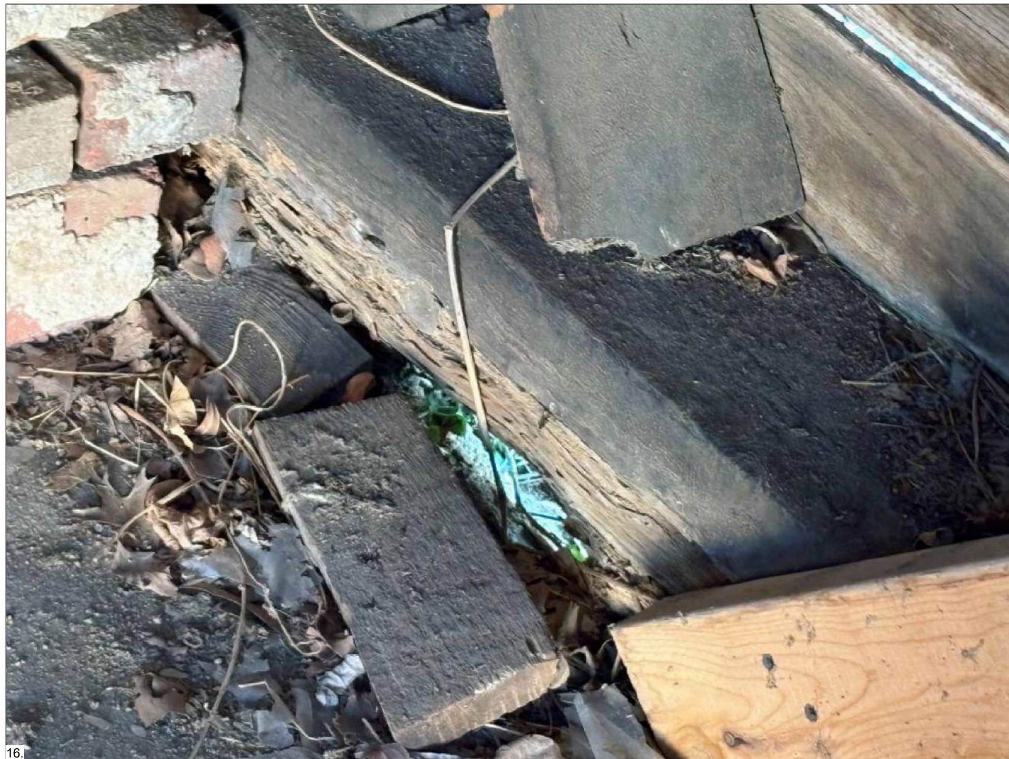
16. SILL PLATE DETAIL SEVERE TERMITE DAMAGE AND ROT CAUSING THE BUILDING TO LEAN
