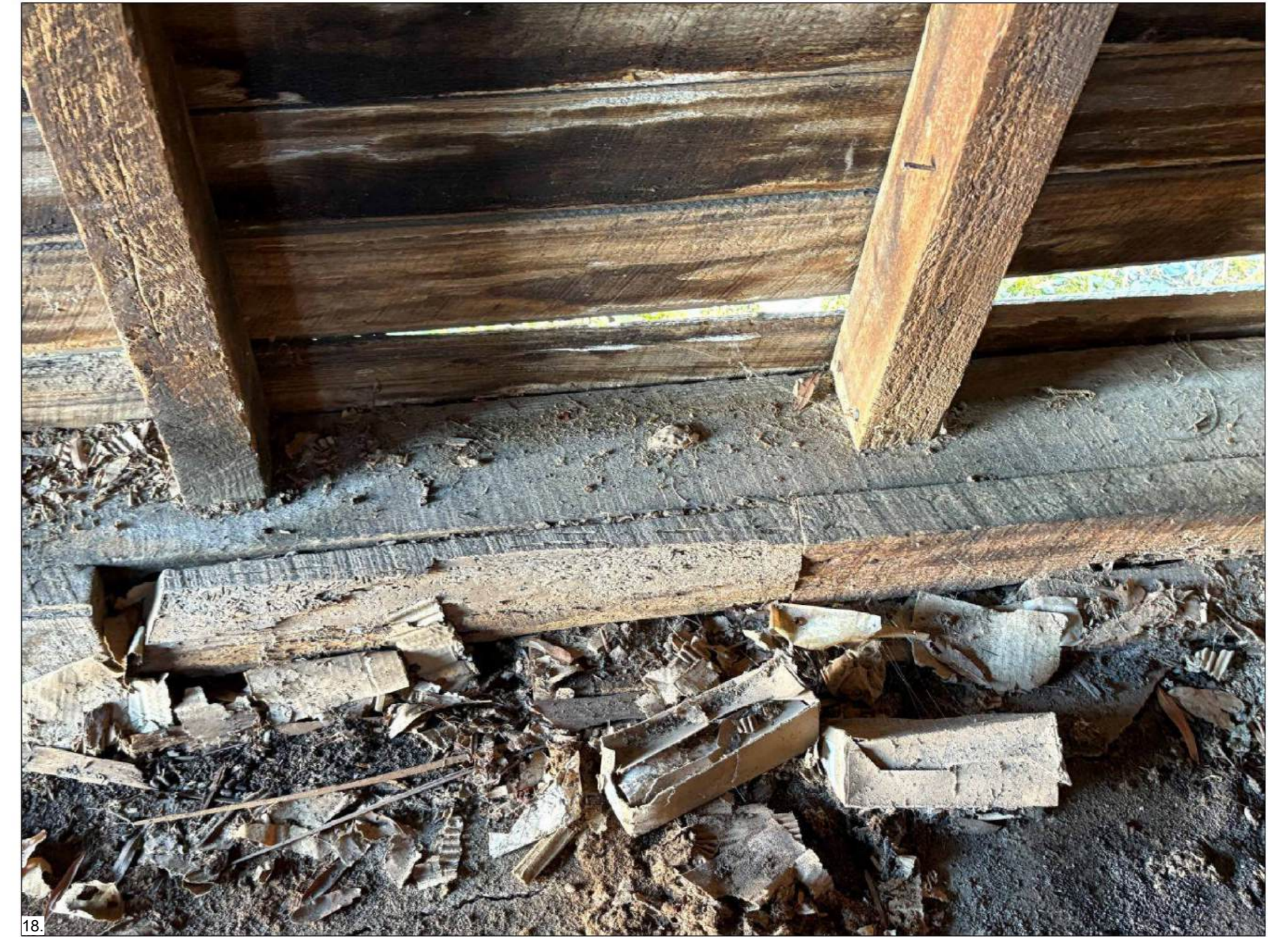
18. SILL PLATE DETAIL VOIDS IN SILL PLATE THAT HAVE BEEN PATCHED WITH WOOD BLOCKING, CONCRETE SLAB NEEDS TO BE REPLACED
