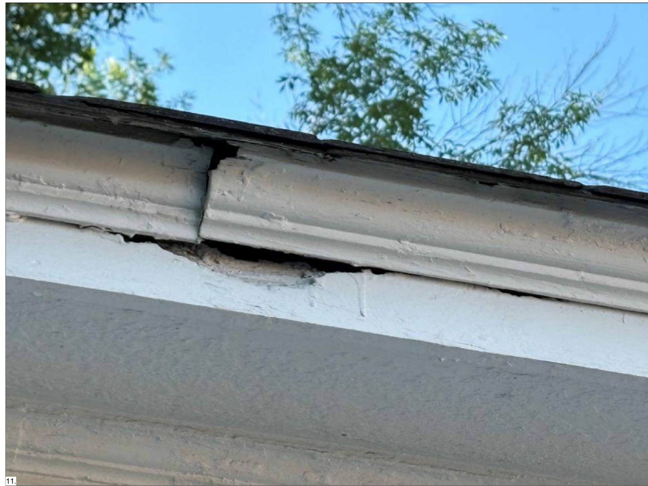
11 CROWN MOLDING DETAIL FACIA AND CROWN MOLDING NEED REPLACEMENT DUE TO EXTENSIVE ROT AND RODENTS
