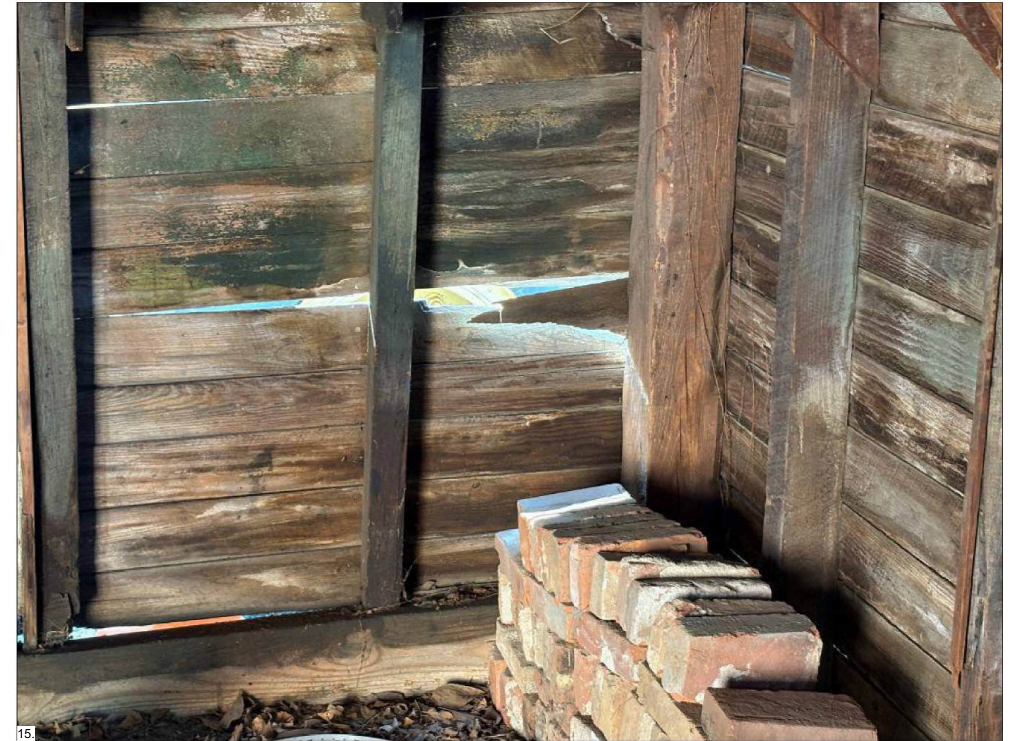
15. INTERIOR SOUTHEAST CORNER SIDING NEEDS REPLACEMENT
