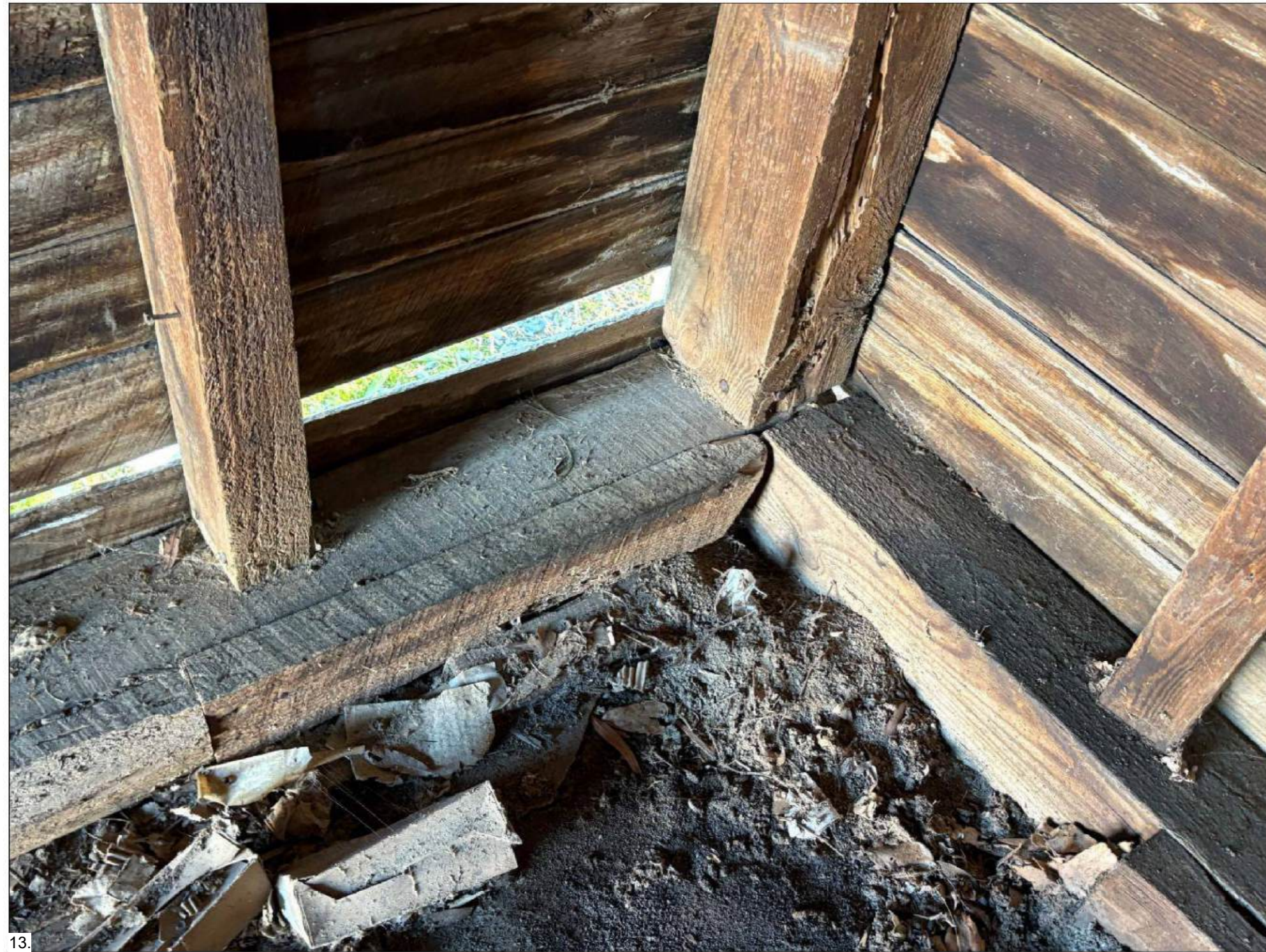
13. INTERIOR NORTHEAST CORNER TERMITE DAMAGE AT CORNER COLUMN AND STUDS, INTERIOR SIDING SHOWS MOLD AND WATER DAMAGE
