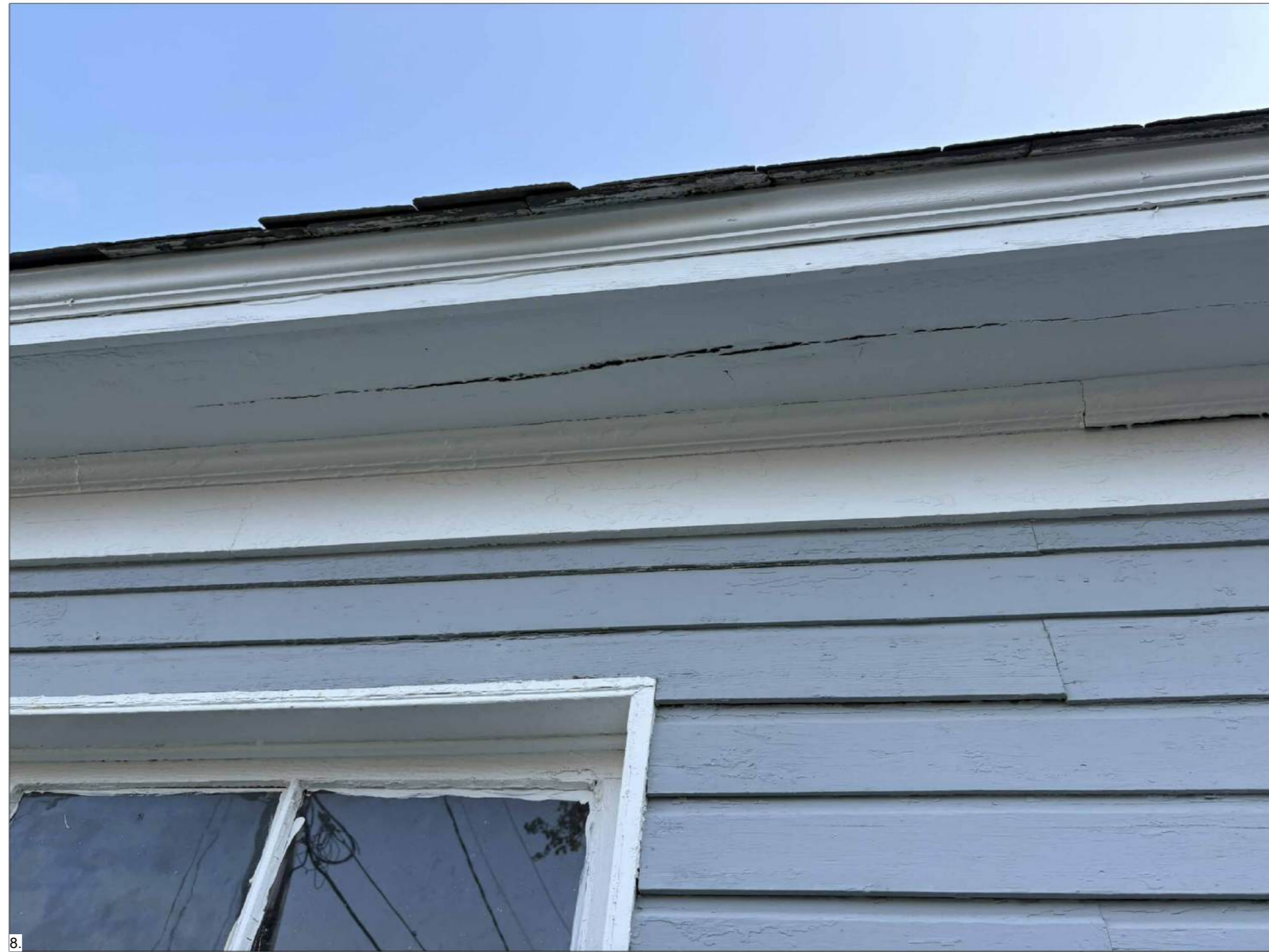
8 SOFFIT DETAIL SOFFIT IS NEEDS REPLACEMENT, EXTENSIVE MOLD AND DECAY
