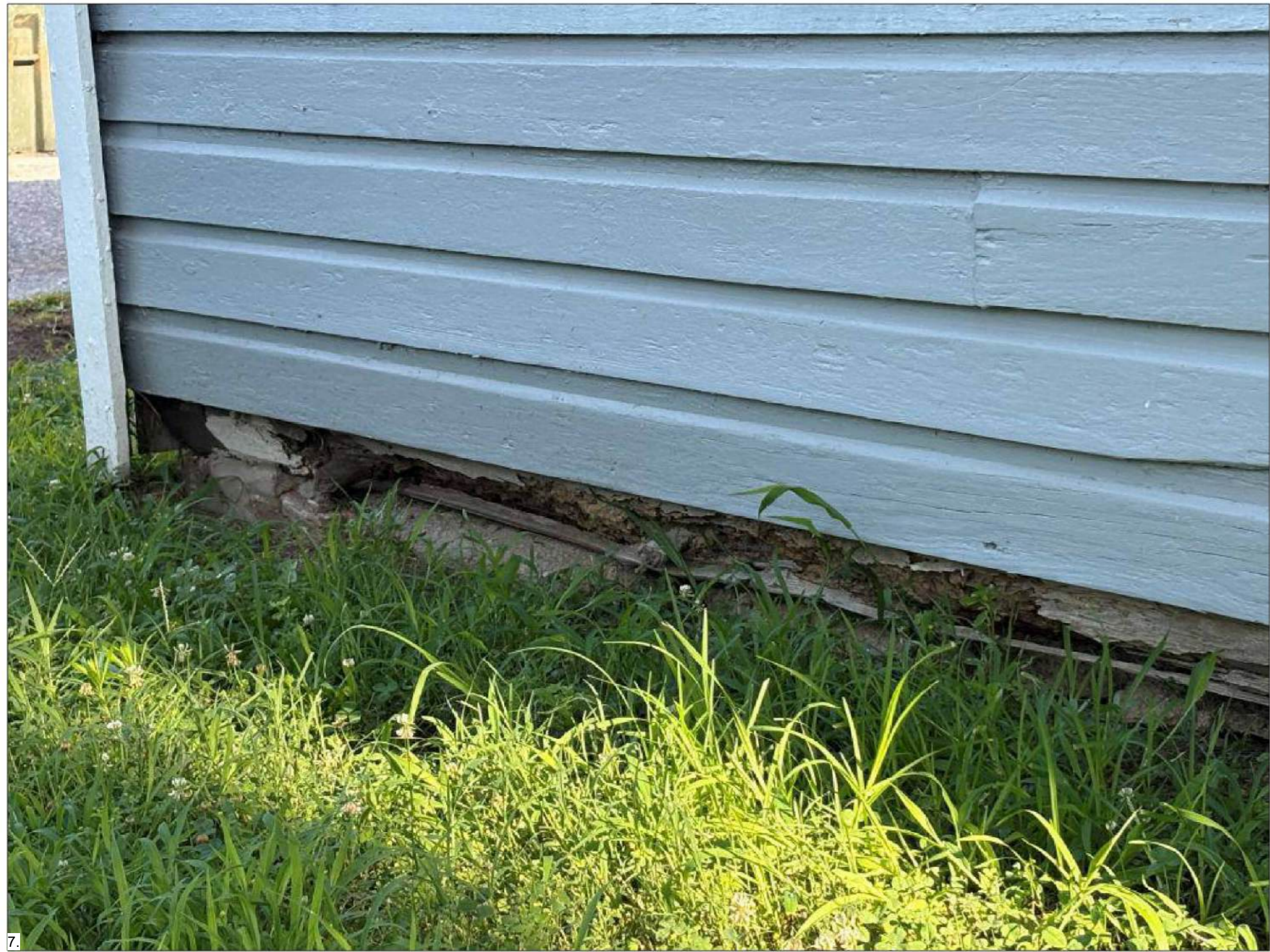
7 SOUTH SILL PLATE SEVERE TERMITE DAMAGE AND ROT CAUSING THE BUILDING TO LEAN, UNCLEAR ABOUT INTEGRITY OF FOUNDATION BUT INTERIOR SLAB HAS CRACKING
