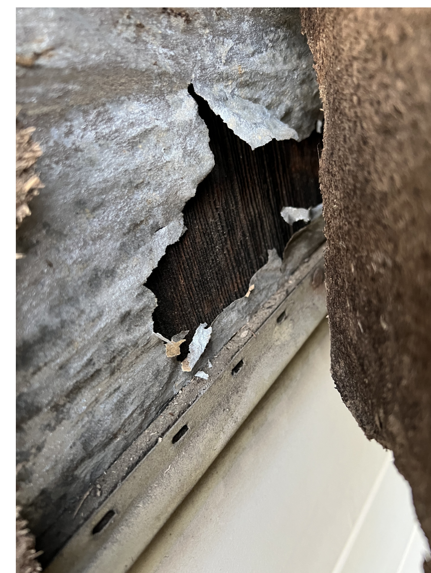
CEDAR SHINGLE UNDER ALUMINUM SIDING
