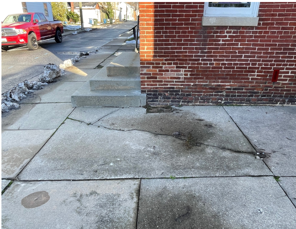
3. Cracked concrete pavement at south stair entry.
