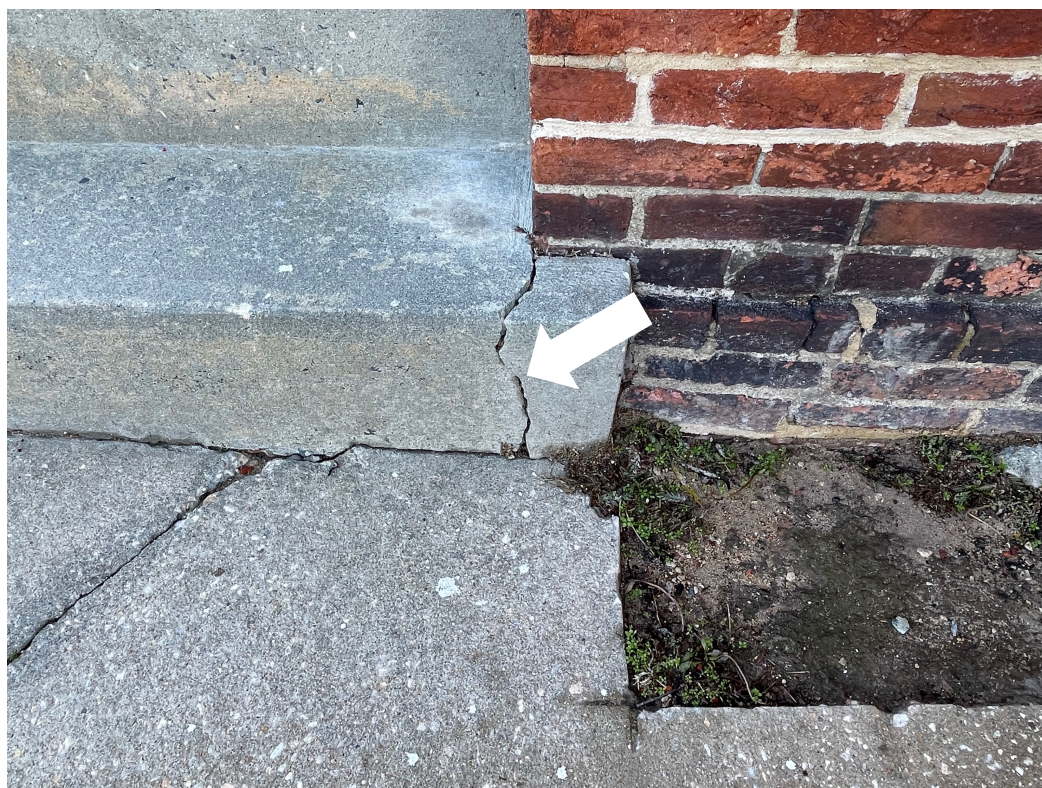
4. Crack in bottom concrete tread at south stair entry.
