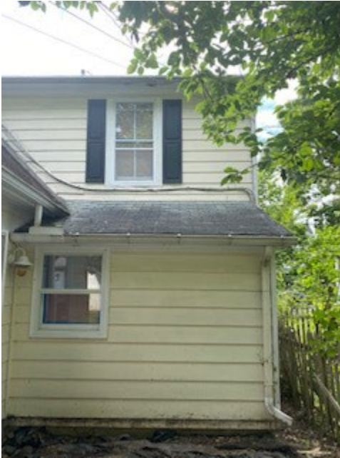
Proposed backyard rooftop location for heat pump unit
