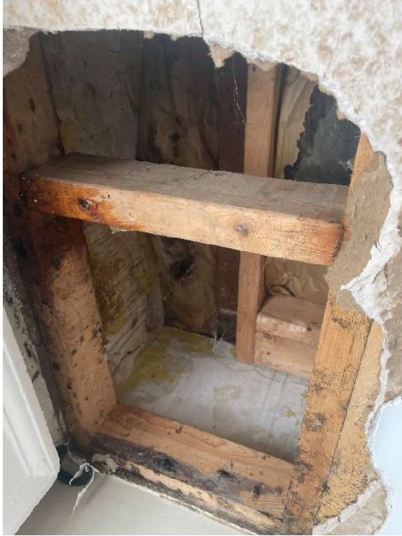
Figure 7: Dangerous mold growth in ceiling caused by rodent-severed condensate drain.
