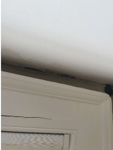
Figure 4: Property damage to drywall and trim caused by rodent-severed condensate drain.
