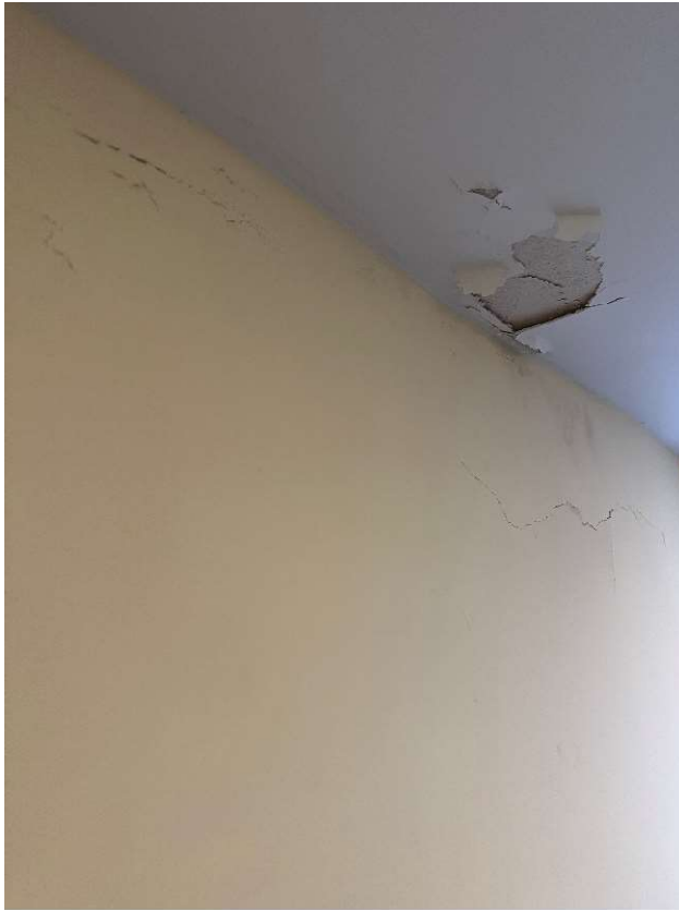
Figure 1: Water intrusion damage in ceiling and wall plaster due to failing roof
