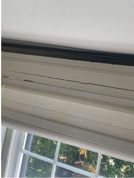
Figure 5: Property damage to window dressing and trim caused by rodent-severed condensate drain.
