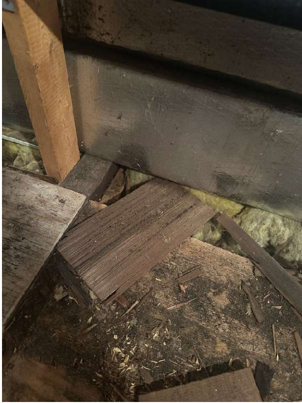
Figure 9: Cedar roofing material found in attic space.
