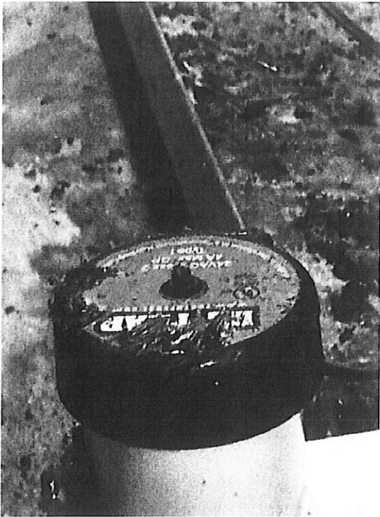
Figure 8: Property damage to new HVAC systems caused by rodent infestation. Note gnawing on equipment as well as destruction of pipe insulation in background.
