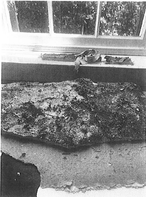
Figure 6: Dangerous mold growth in ceiling caused by rodent-severed condensate drain.
