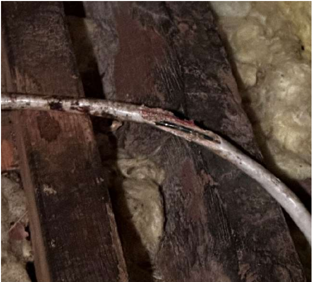
Figure 2: Life safety hazard caused by rodent infestation due to failing roof.
