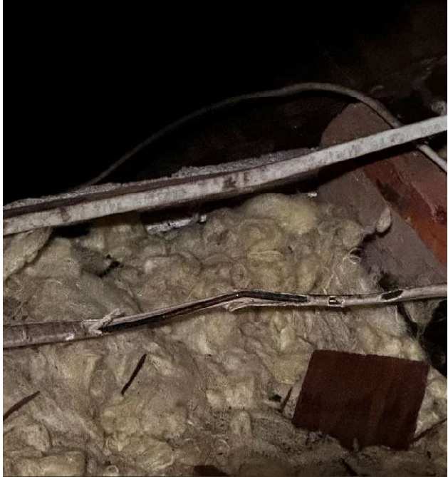
Figure 3: Life safety hazard caused by rodent infestation due to failing roof.
