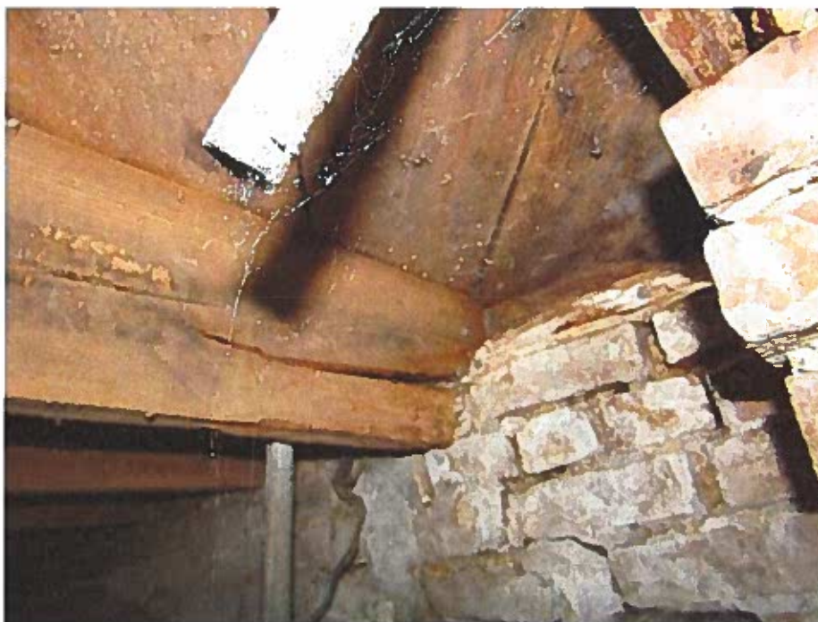
PHOTOGRAPH 16 Rotten floor joists and deteriorated brick/mortar in the crawlspace.
